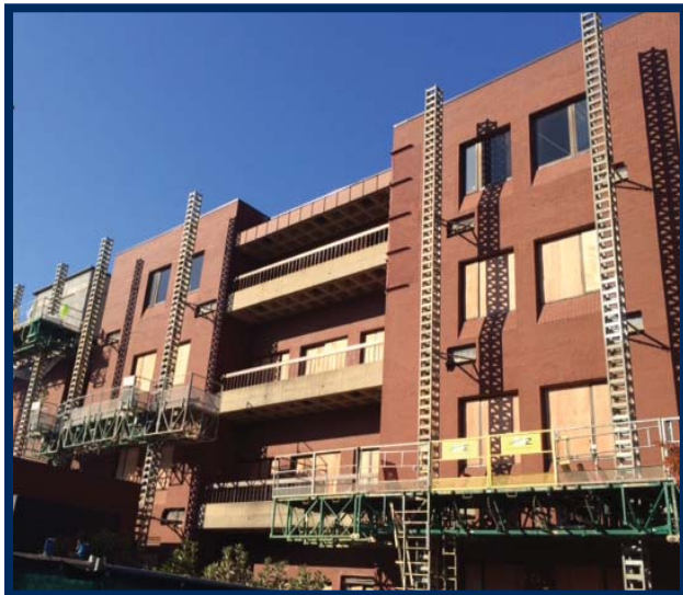
South Elevation - Scaffolding and Work Platforms Installed for Brick and Window Removal
