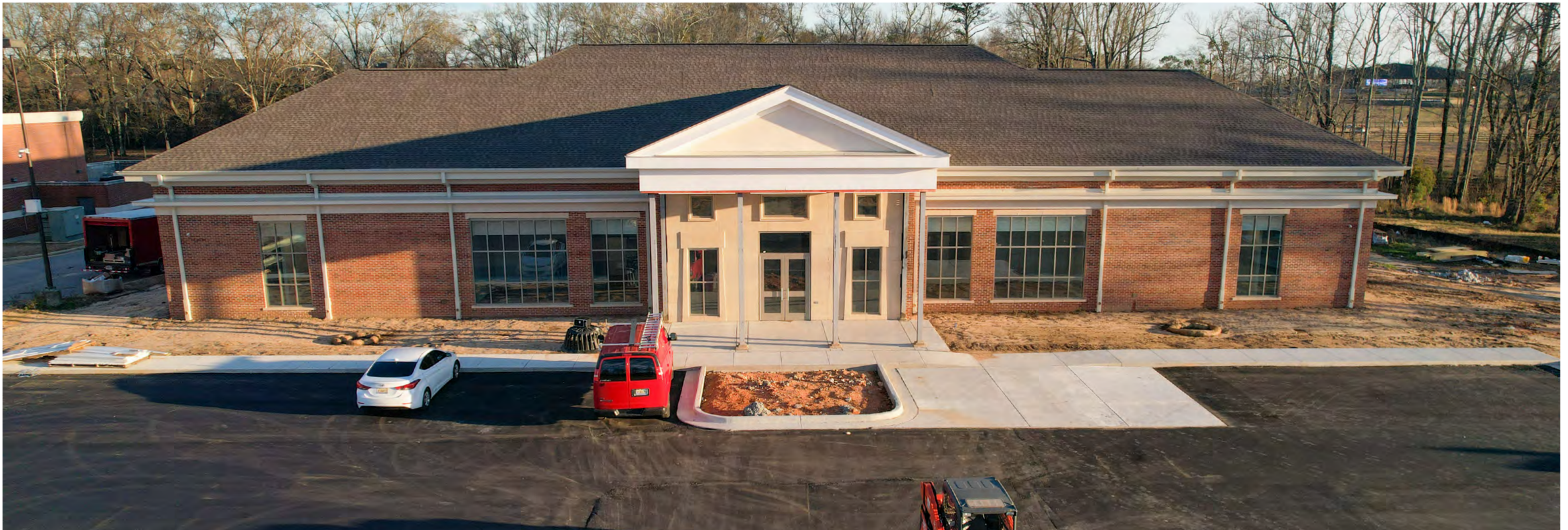
The main entrance to the facility is coming together. Hardscape installation is wrapping up and landscape installation will start soon.
