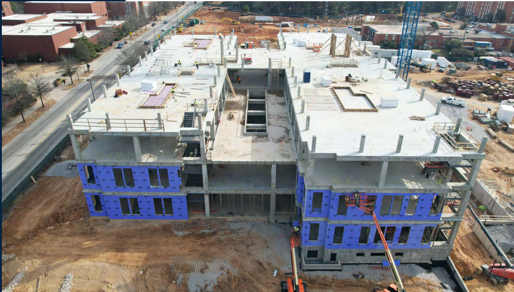
The exterior barrier is being placed on the first and second floors.
