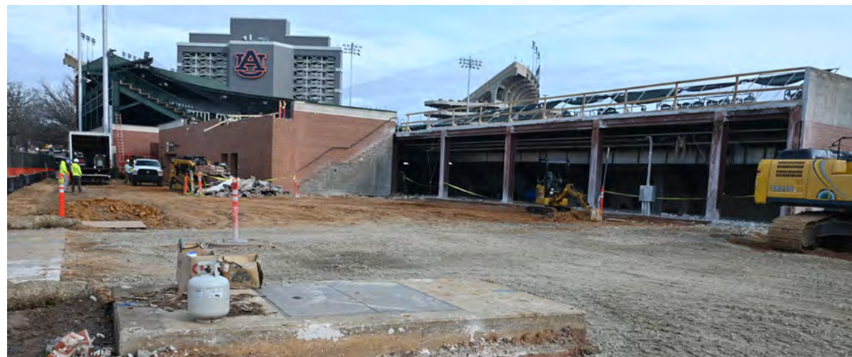
Demolition of a brick wall behind the first base line seats in preparation for the new kitchen in the First Base Club.
