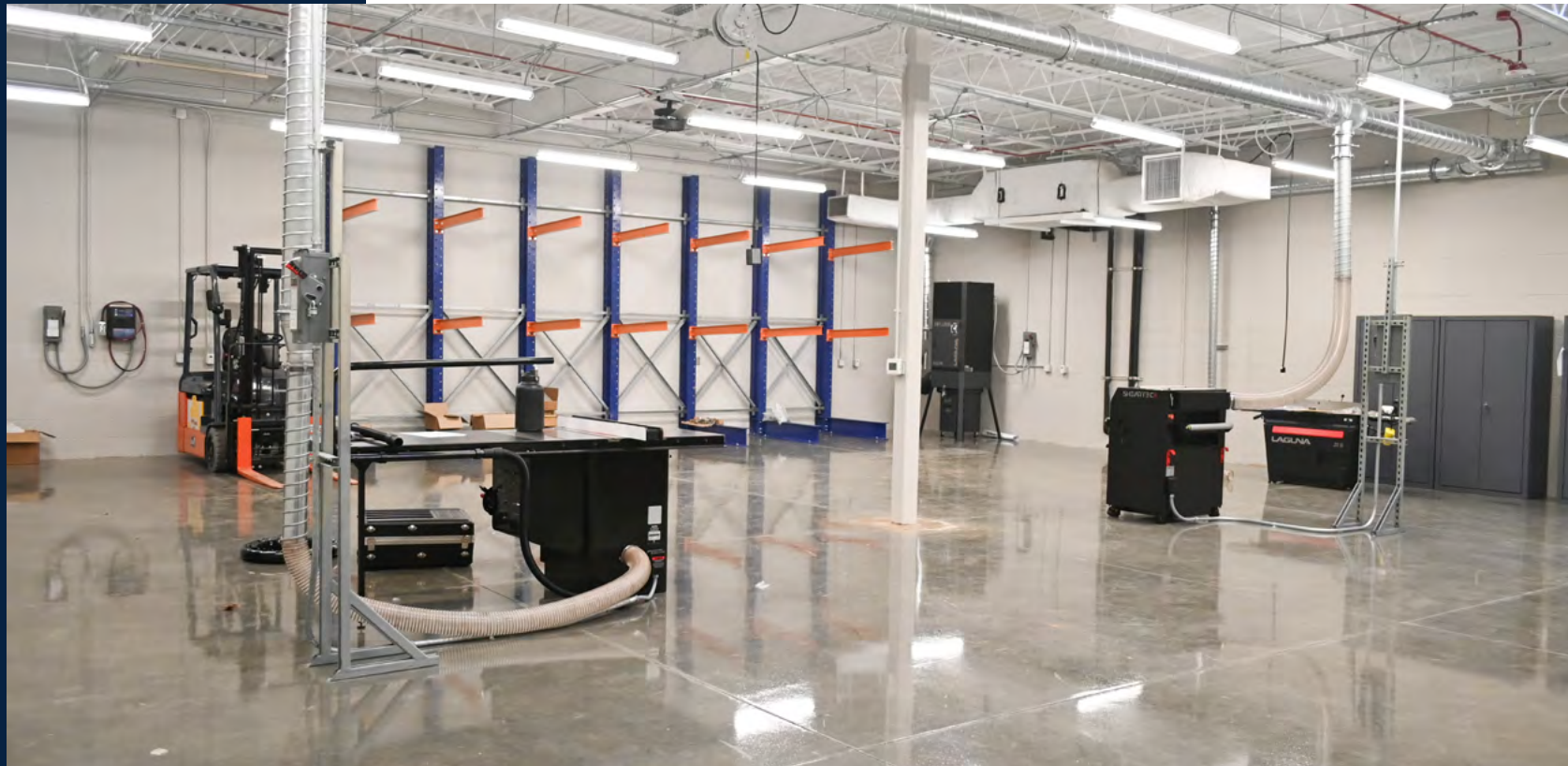
The CADC Mass Timber Research Initiative space is complete and ready for use.
