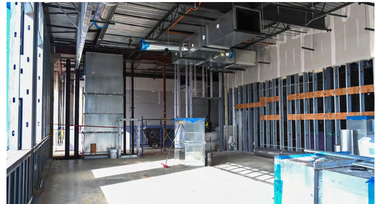
In-wall and overhead mechanical, electrical and plumbing systems installation continues in this new lab room.
