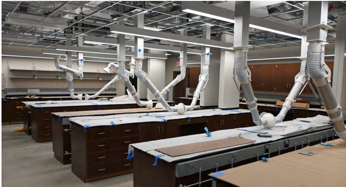
Lab installation is nearing completion with the mechanical, electrical and plumbing installed.
