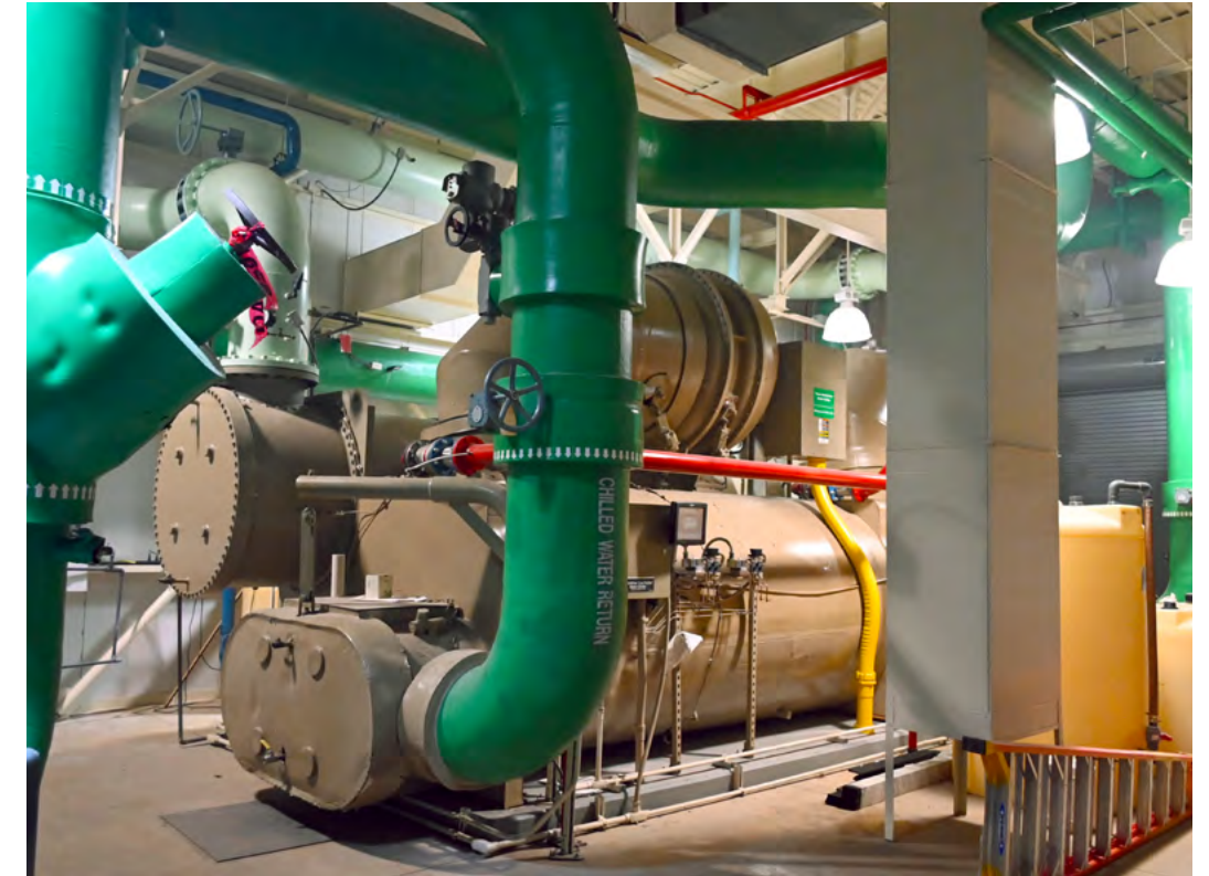
This existing chiller will remain in place.
