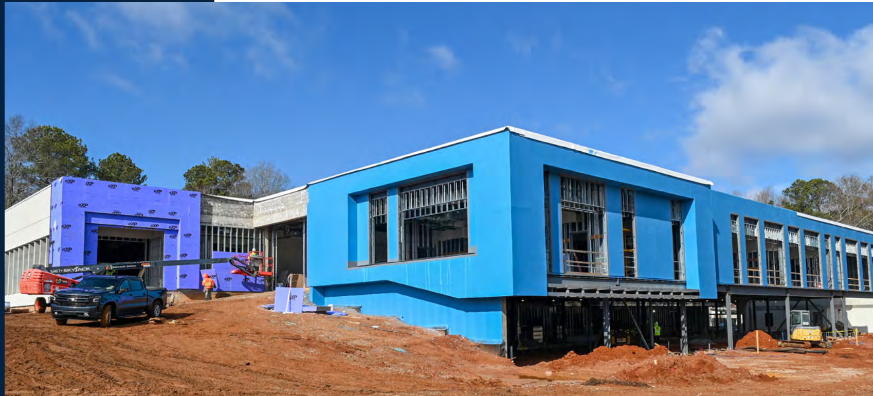
A protective waterproof barrier has been installed on the outside of the building.
