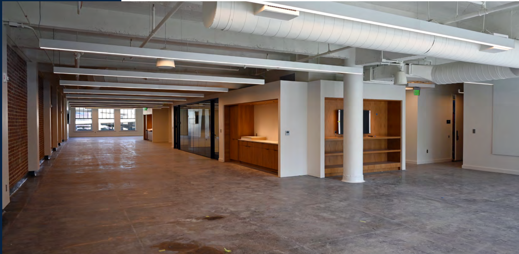
Collaborative spaces and small meeting rooms on the sixth floor are waiting for furniture installation following completion of telecommunication equipment installation.
