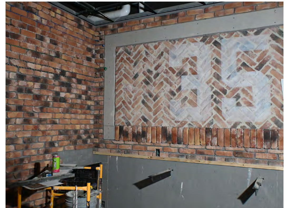
Brick finishes are going up for the interior Hall of Fame Club space.
