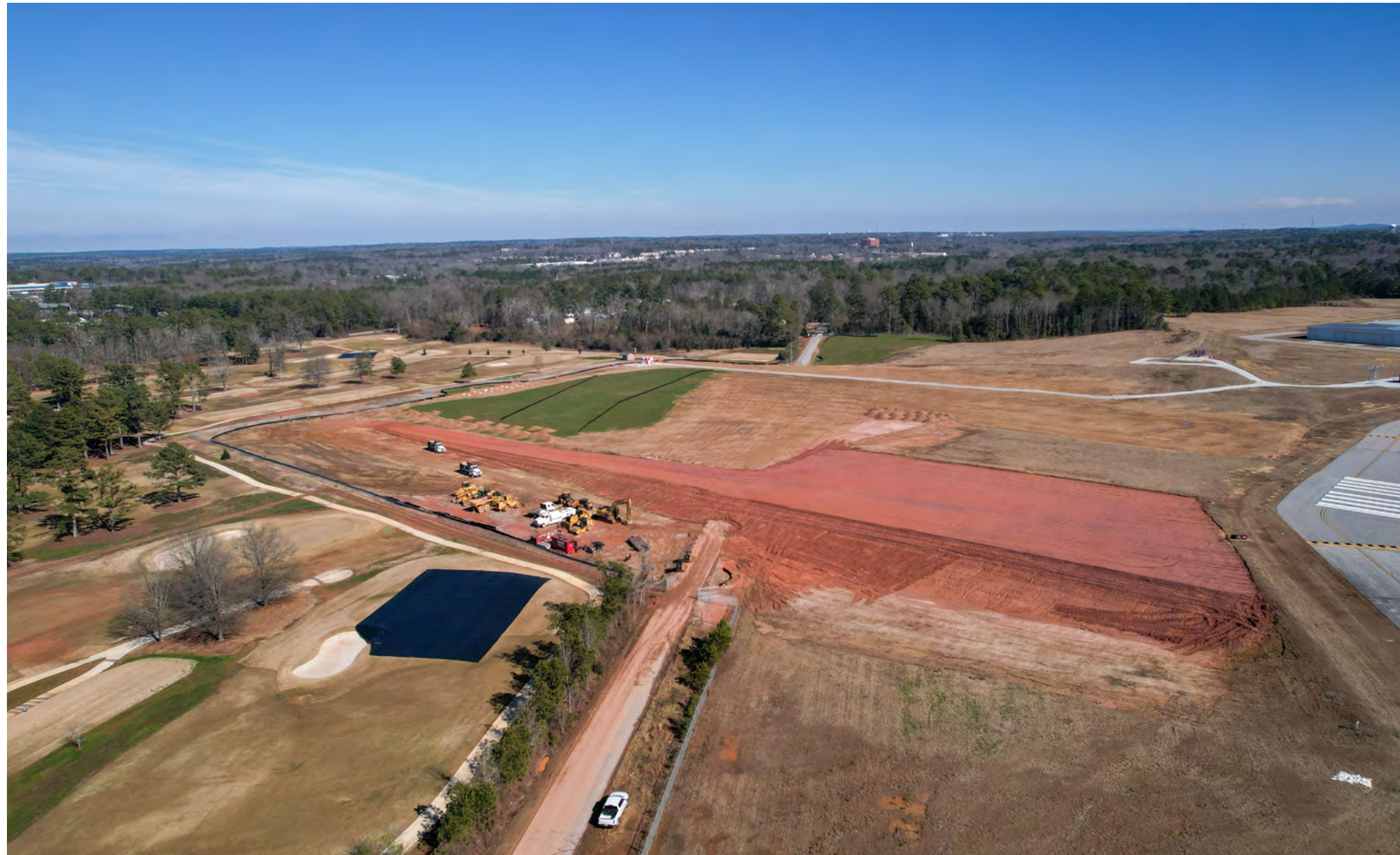
Dirt fill continues to be hauled in and placed. Site preparation for the new localizer antenna platform is underway.
