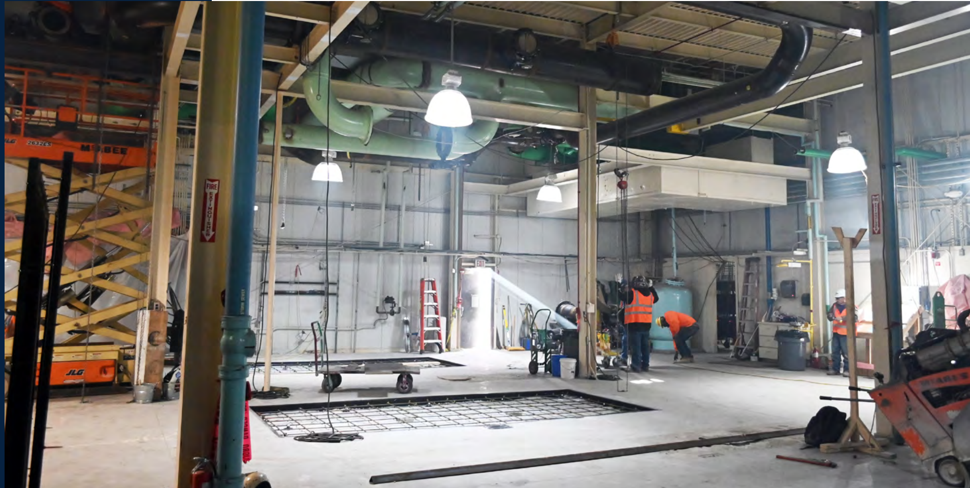
The chiller equipment room is being prepared to pour concrete bases for the new chillers.
