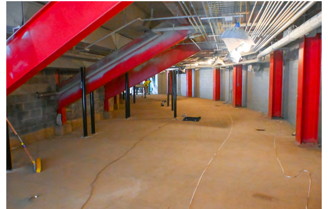
The corridor entry to the field level seats is ready for paint and furnishings.
