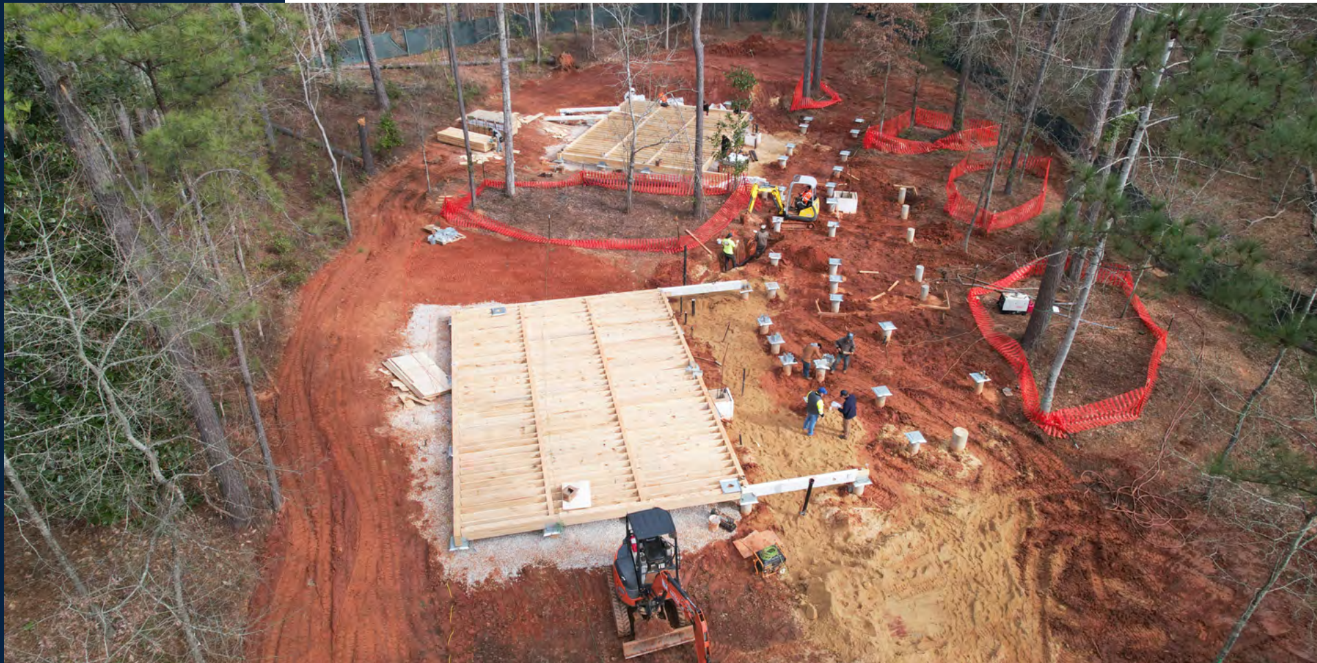
An aerial photo illustrates where concrete foundations have been poured for the new building.
