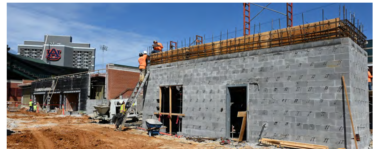
The horizontal beam is being formed on top of the first level.
