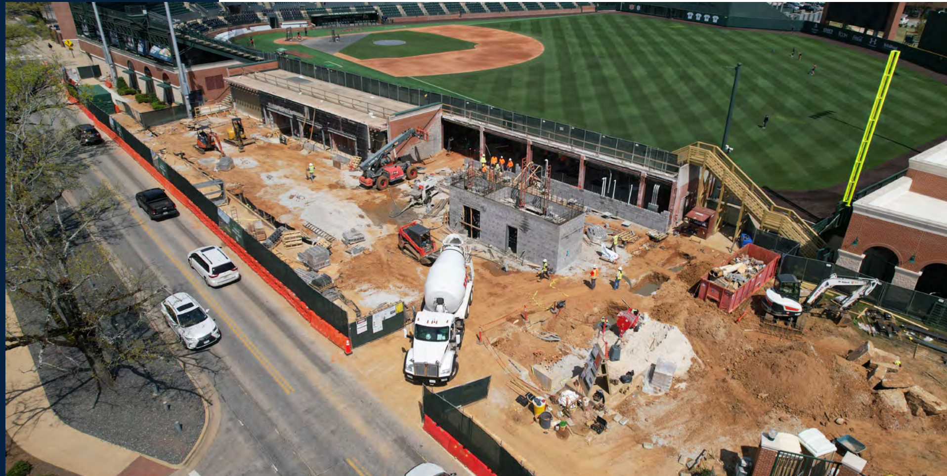
Overview of the First Base Club. Foundations are complete before the structural steel arrives in early April.
