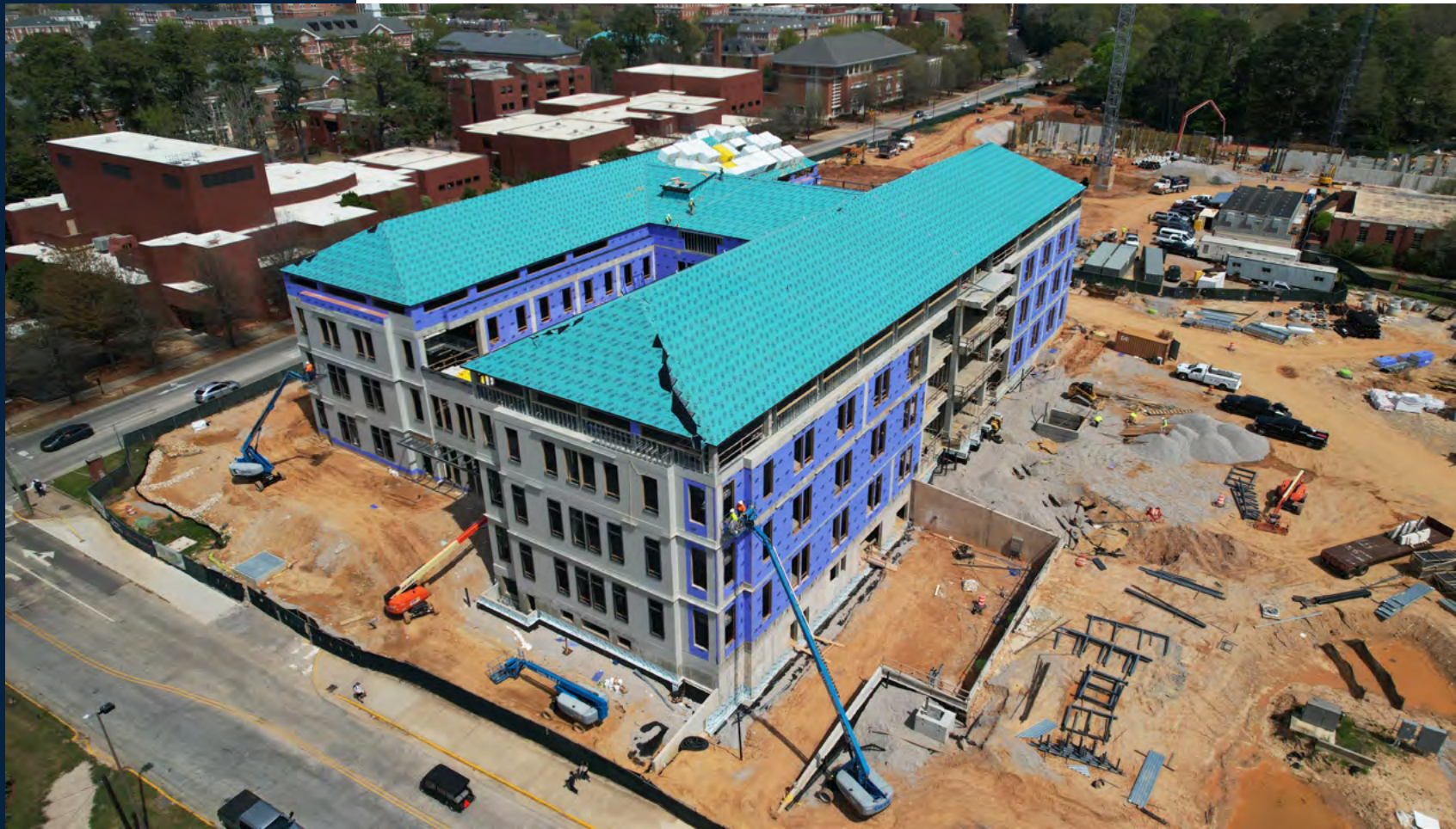
The building's roof decking is in place, while installation of the protective waterproof barrier is ongoing.
