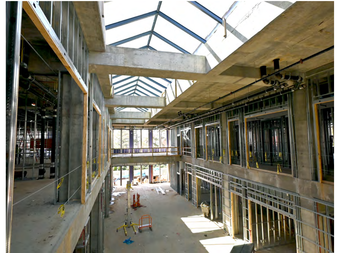
The skylight, which allows natural light into the central atrium space, is complete.
