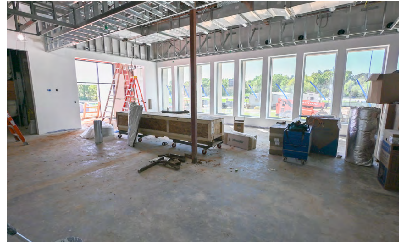
Overhead mechanical installation nears completion in the lobby of the science lab building.
