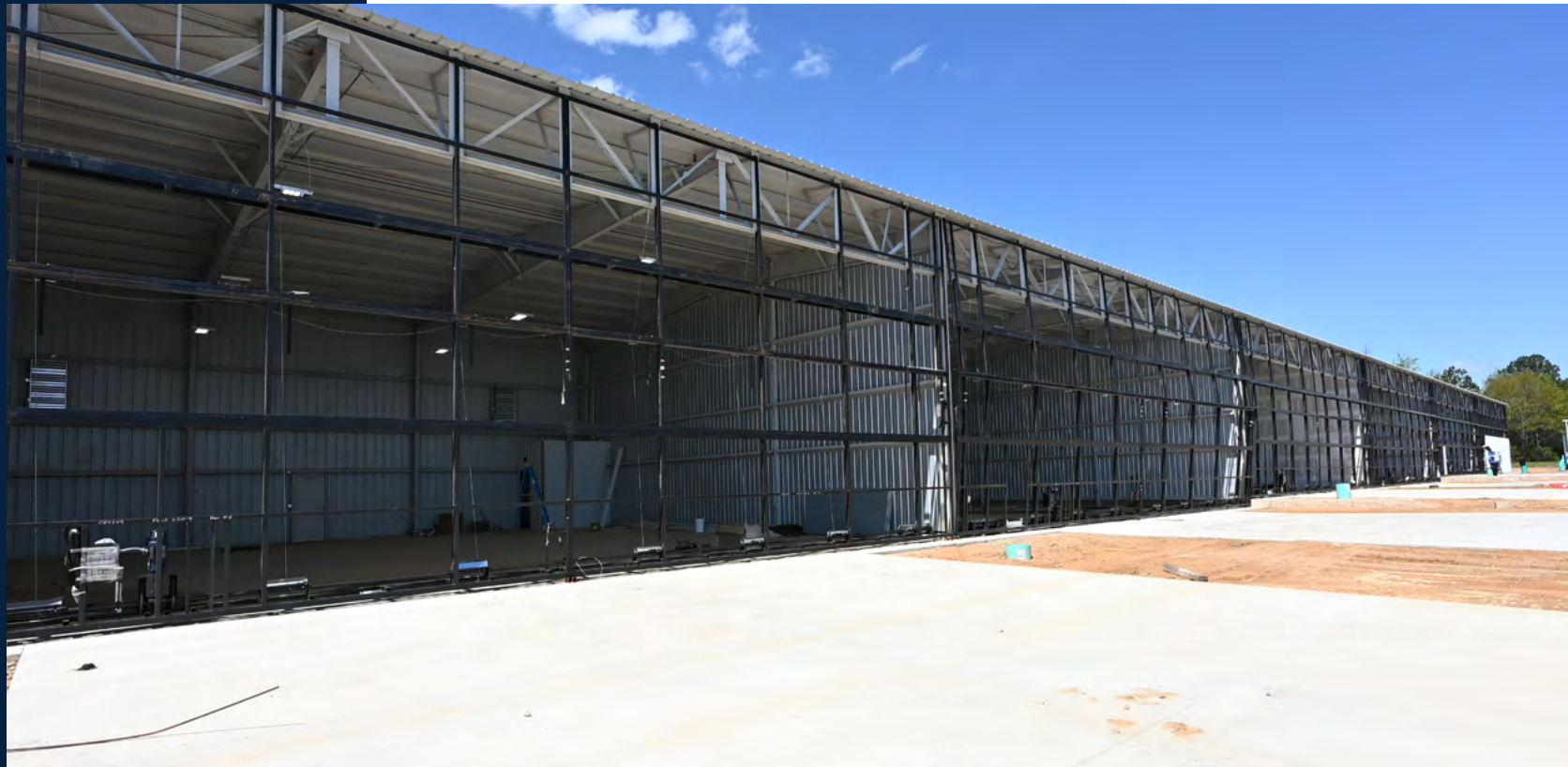
Mechanical hangar door frames are in place. Next steps include installation of the metal door coverings.
