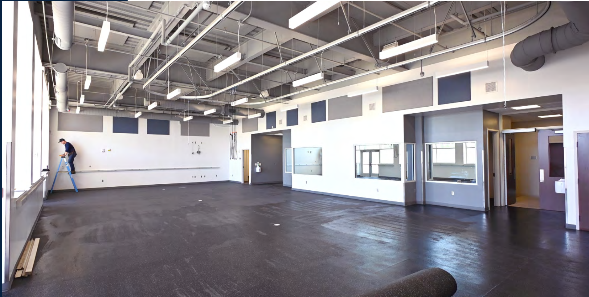
Installation of flooring and final paint is taking place in the School of Kinesiology's Doctor of Physical Therapy clinic space in the Kinesiology Building.
