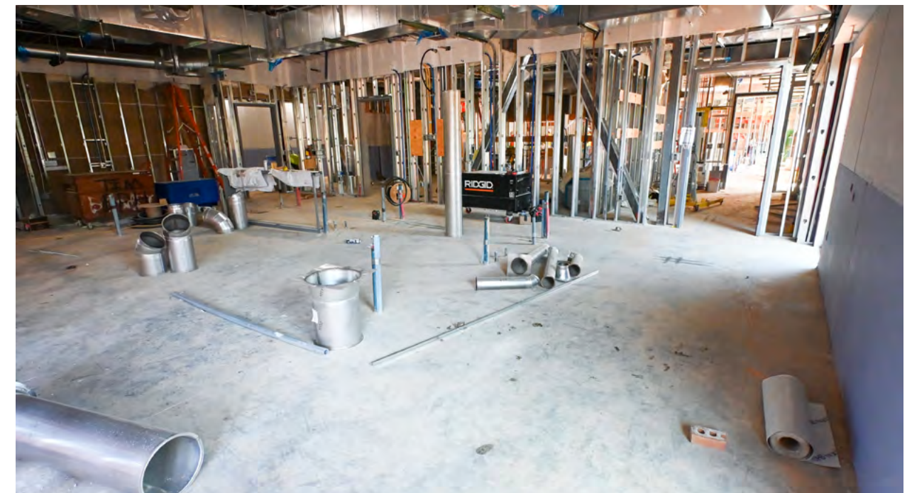
Mechanical and electrical work continues in the walls and overhead in the ground floor laboratory.
