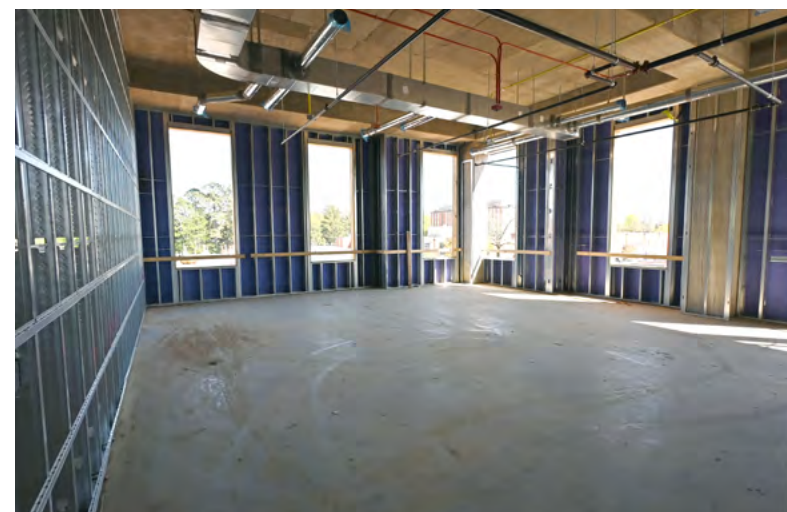
Framing is complete for this second floor active learning classroom that will have a dual function as a computer lab.
