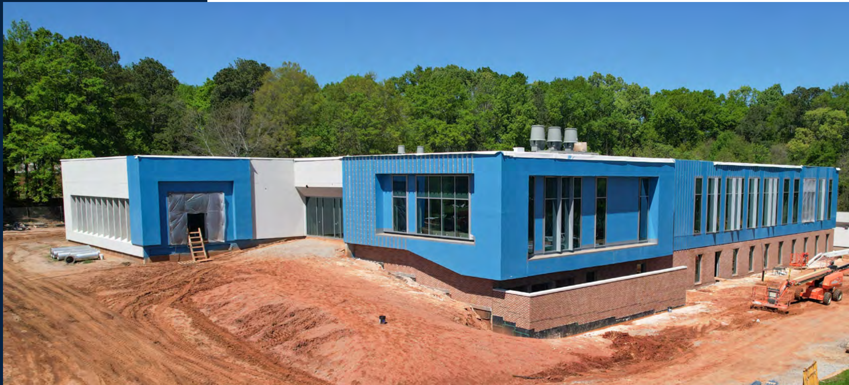
The building facade is nearly complete. Metal panels are being manufactured for installation in the blue areas in mid-June.
