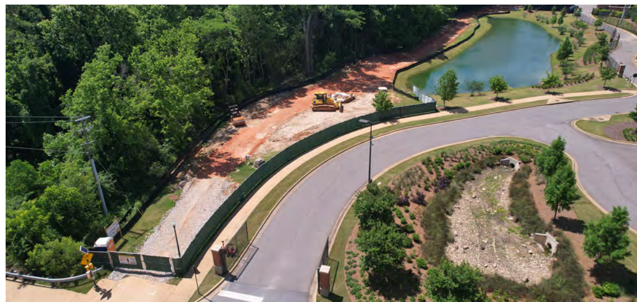
The Lem Morrison Drive entrance to Phase III is being prepared for construction of the 10-foot wide concrete multi-use pathway.
