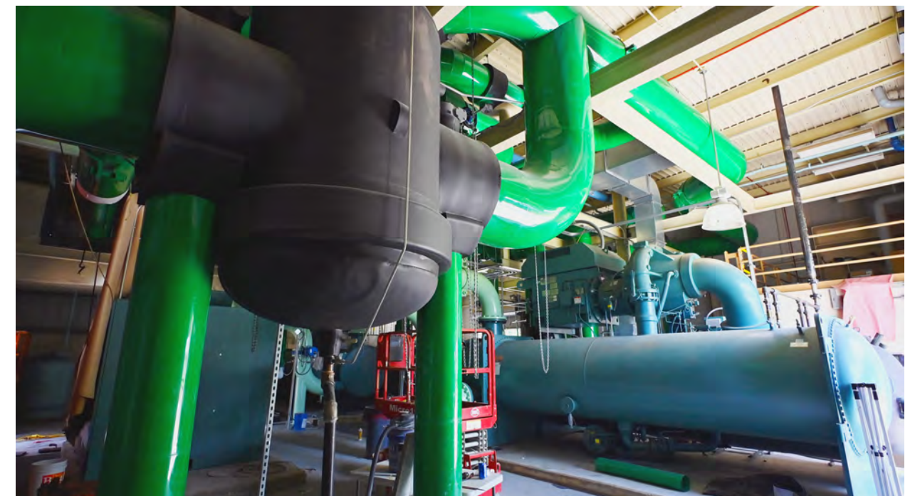
The new piping system will handle the higher water yield of the new chillers.
