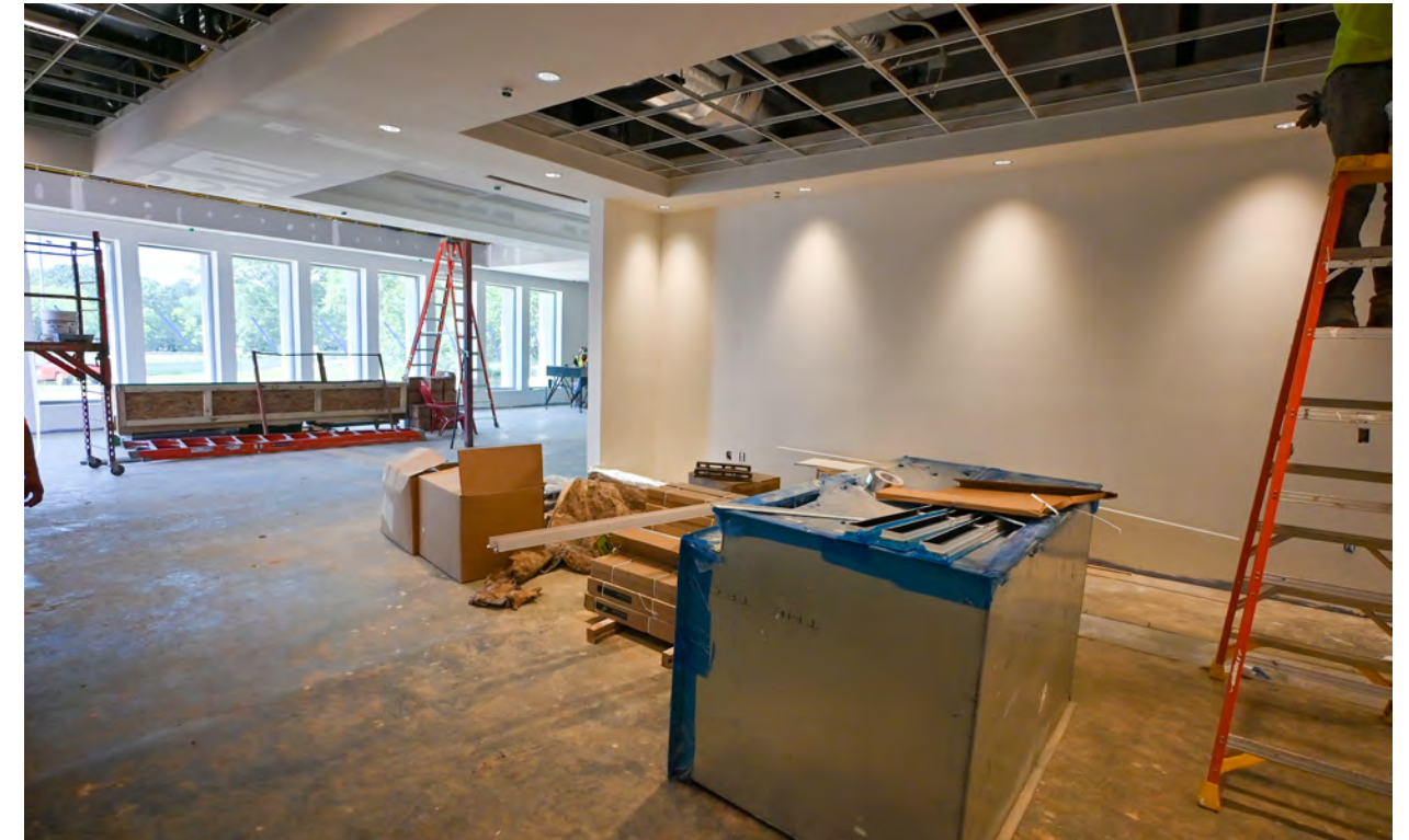
Walls are being primed and painted in the lobby, while mechanical systems are being installed overhead.
