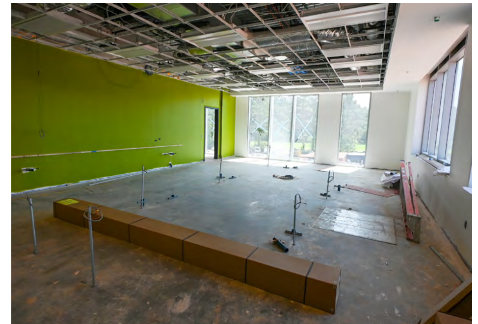
Freshly painted walls set the backdrop for this laboratory classroom with cabinetry, ceiling tile and flooring installation to begin soon.
