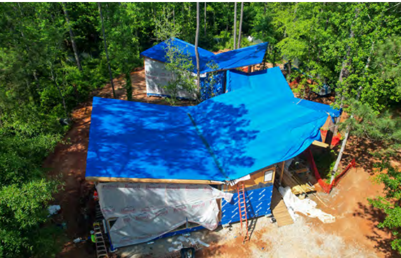
Aerial view of the Environmental Education Building as it progresses toward completion.
