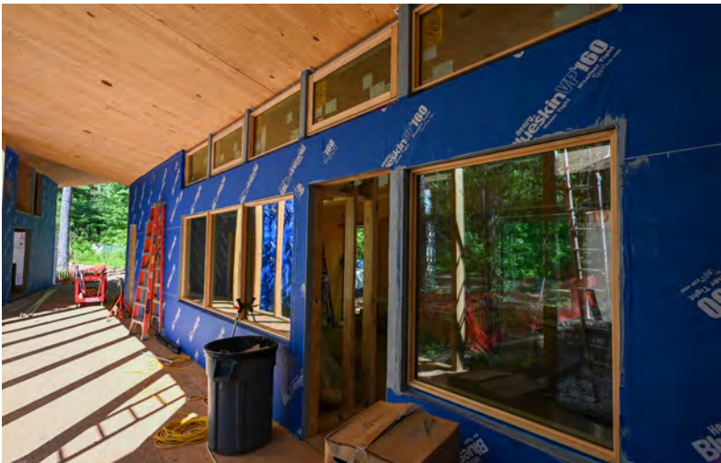
Main structure pieces are being installed and are ready for final finishes.
