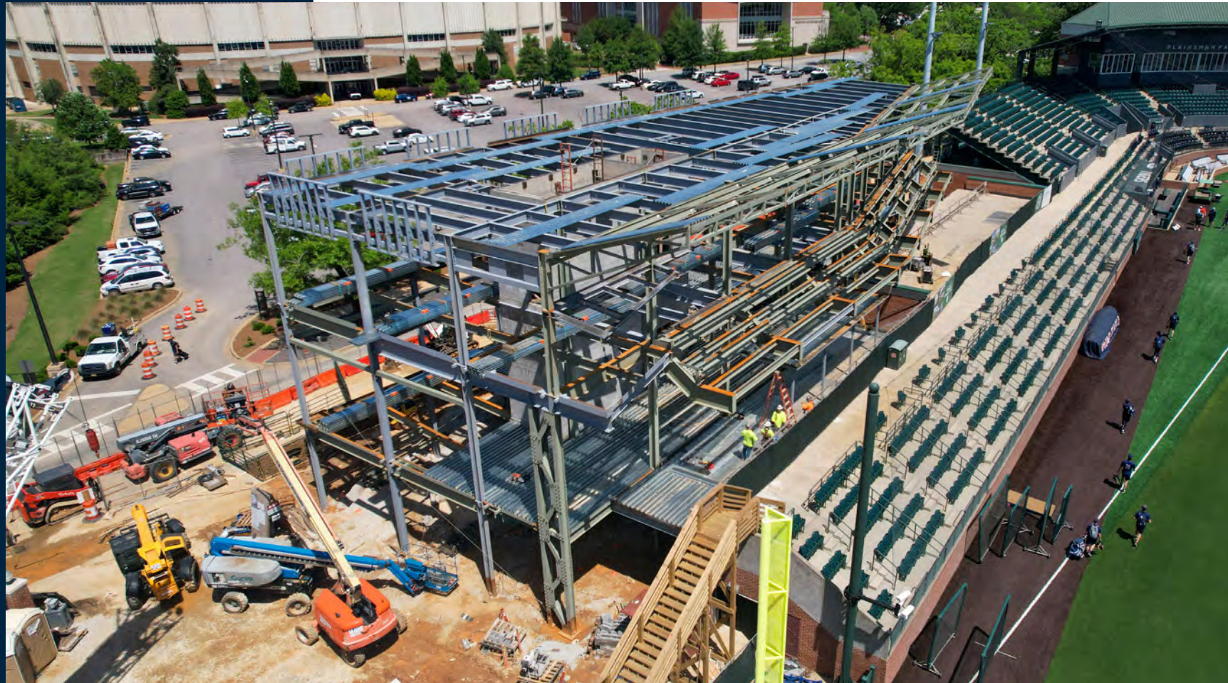
The three-story steel structure for the first base line expansion nears completion.
