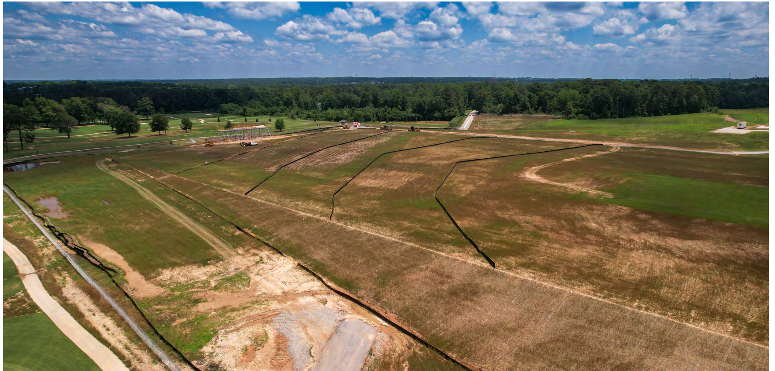
The Auburn University Regional Airport Runway Safety Extension Project is complete. Storm water silt fences will remain until grass is established.
