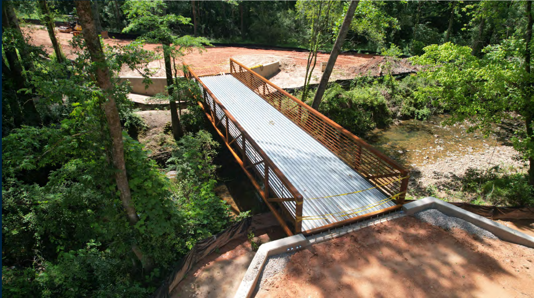
The bridge has been installed across Parkerson Mill Creek. View installation video.
