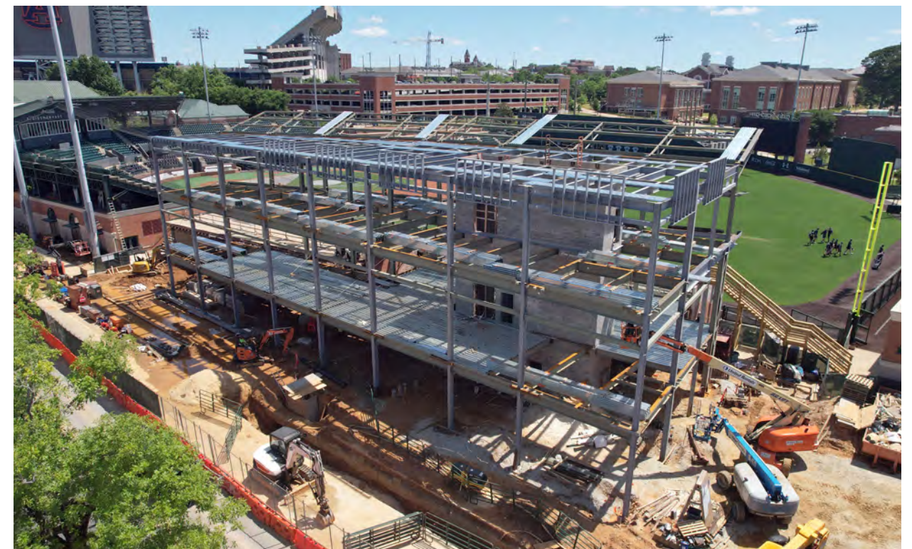
This view from Donahue Drive shows where steel decking is being installed for the first steps of floor installation on the second level.
