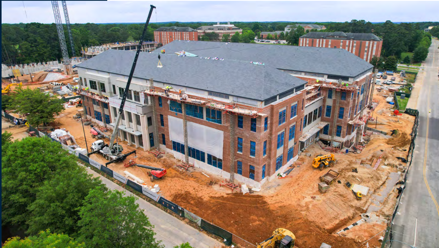
Brick work and roofing continues on the exterior of the College of Education building.
