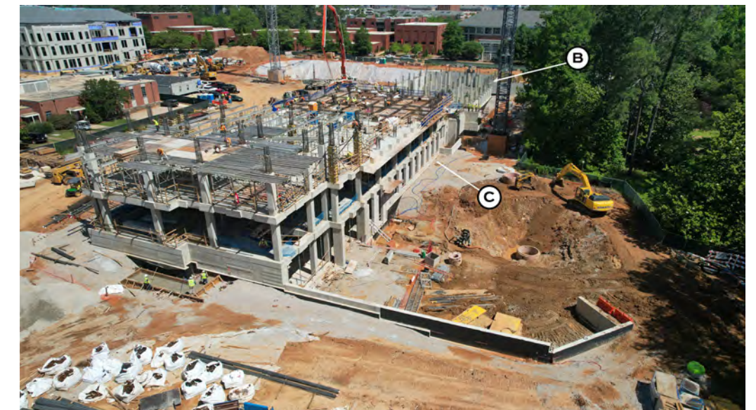
View of Building C from the Southeast. Formwork for the second floor is in progress.
