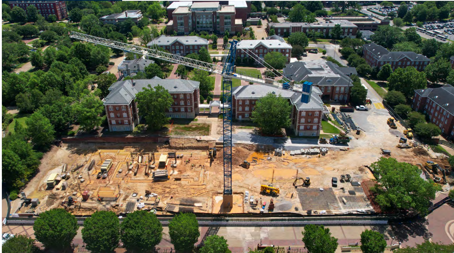
Columns, walls and foundation work is underway at the New University Student Housing site.
