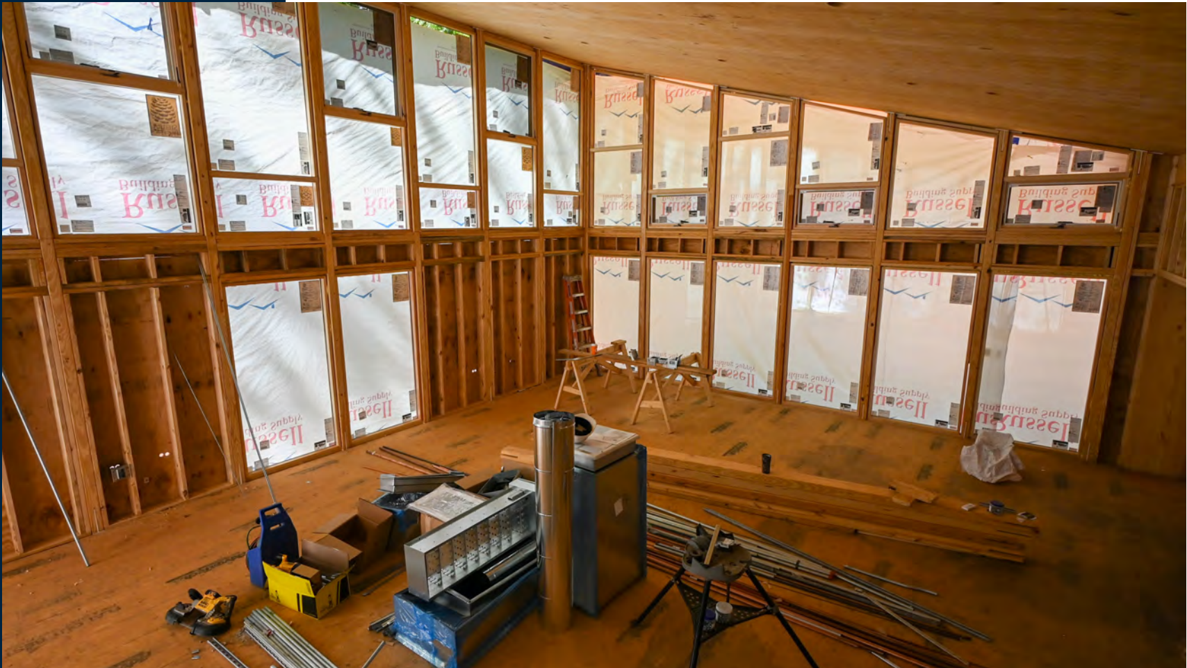
Windows have been placed within the classroom areas of the Cross Laminated Timber (CLT) structure.
