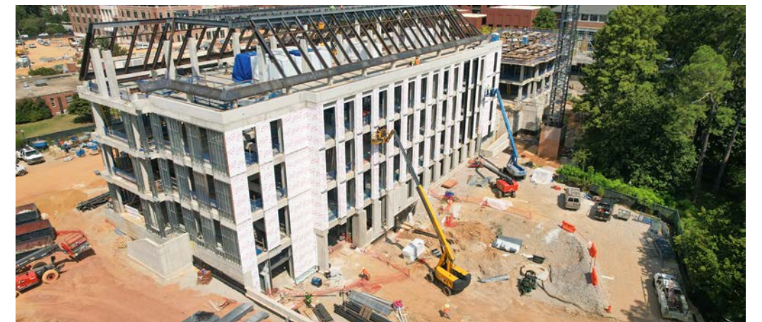
External wall framing continues of the east and south sides of Building C.
