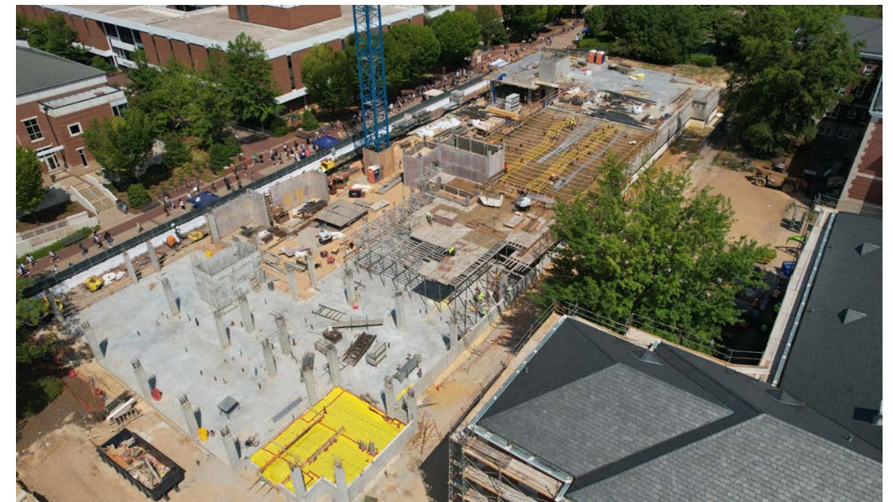
Concrete foundations and columns are being installed on the Quad Drive side of the project.
