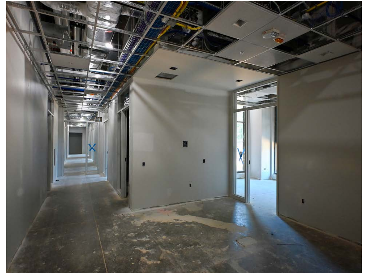
The office space on the second floor is ready for ceiling tile and flooring installation.
