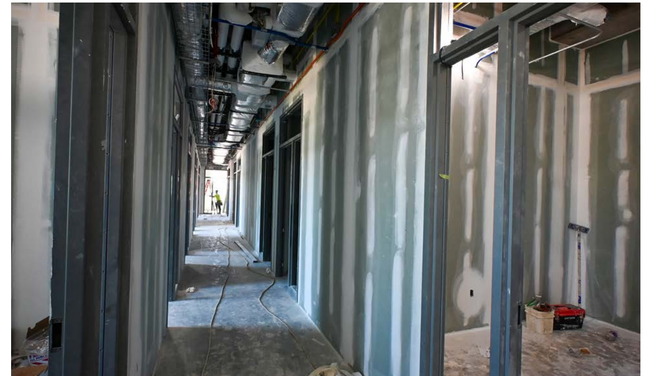
Drywall installation nears completion on the third floor with walls being prepped and primed for the first coat of paint.
