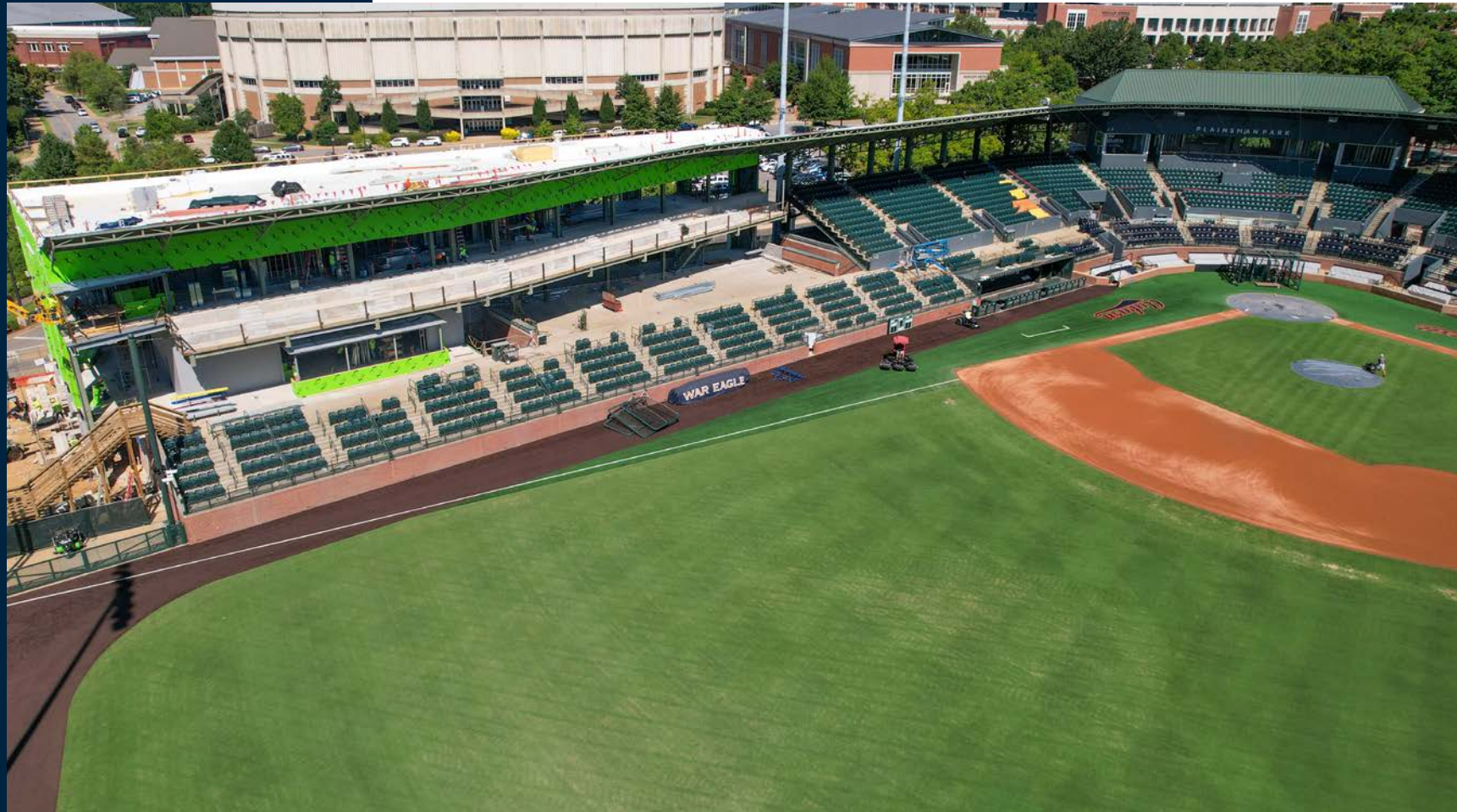
An aerial view of the three-story addition along the first base line.
