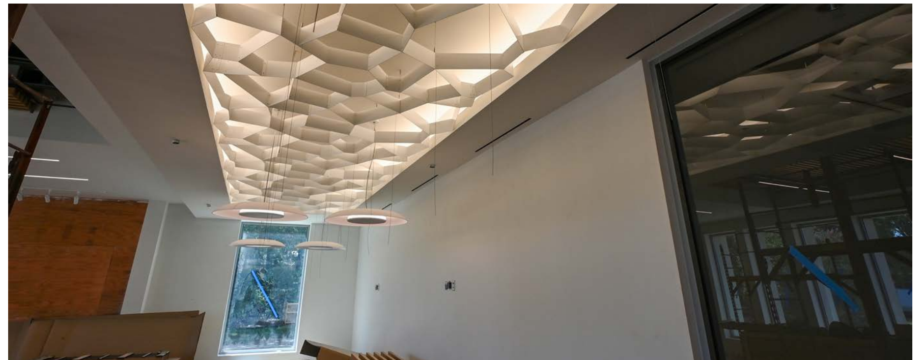
The decorative lobby ceiling and light fixtures are installed, which will welcome visitors into the main public space.
