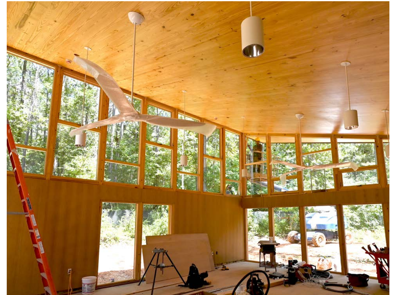
Indoor fans and lighting have been installed within the classroom areas of the structure.
