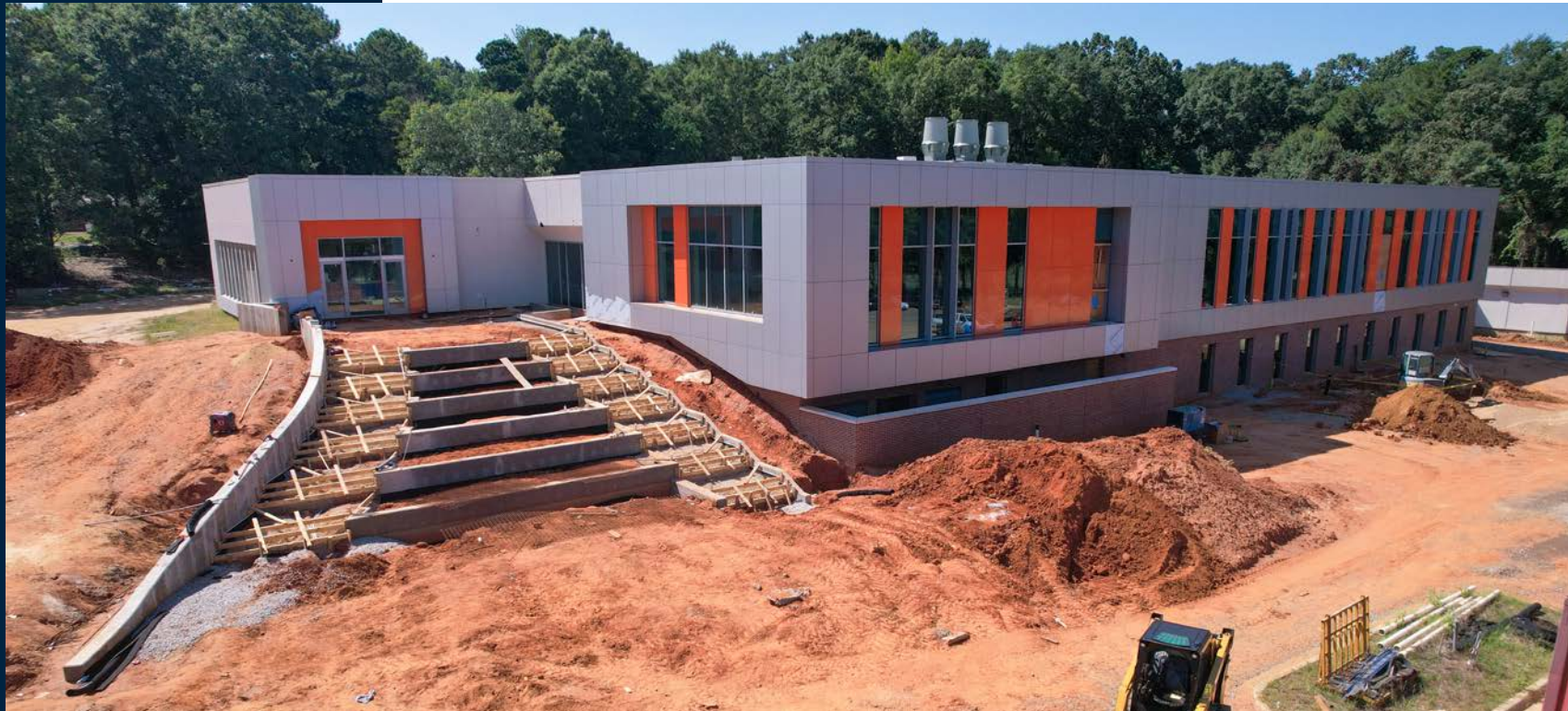
The main entrance steps are being carefully formed and will soon be ready for concrete, marking a significant step towards the completion of the exterior.
