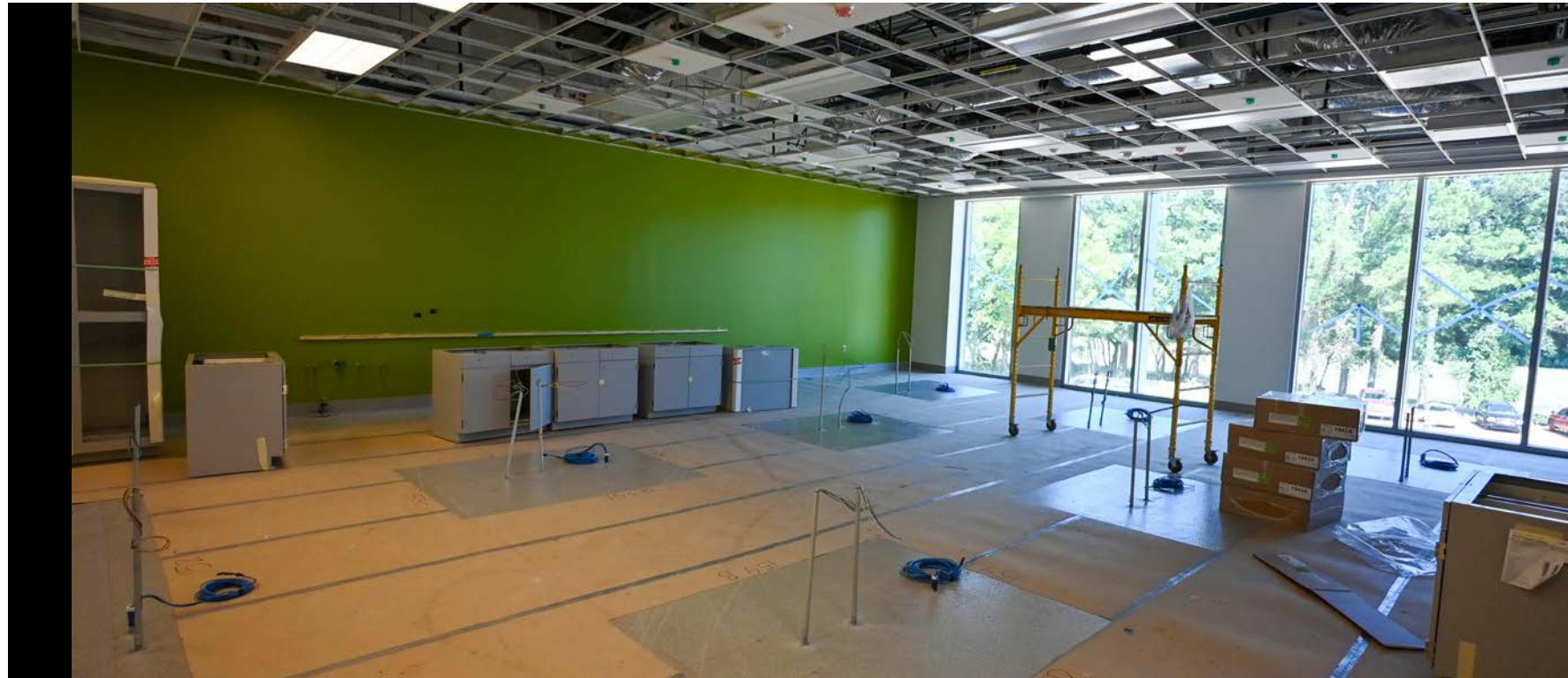
Casework installation has begun in this lab with electrical and plumbing lines stubbed up through the floor, ready to be connected.
