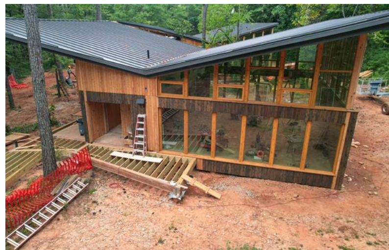
Tempered glass has been installed along the outside of the main structure.
