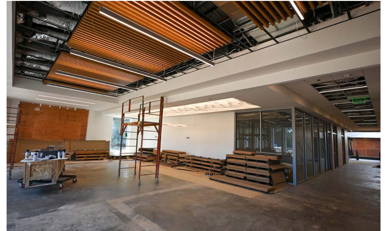
New lighting illuminates the lobby as the workers install the wood slatted ceiling panels.
