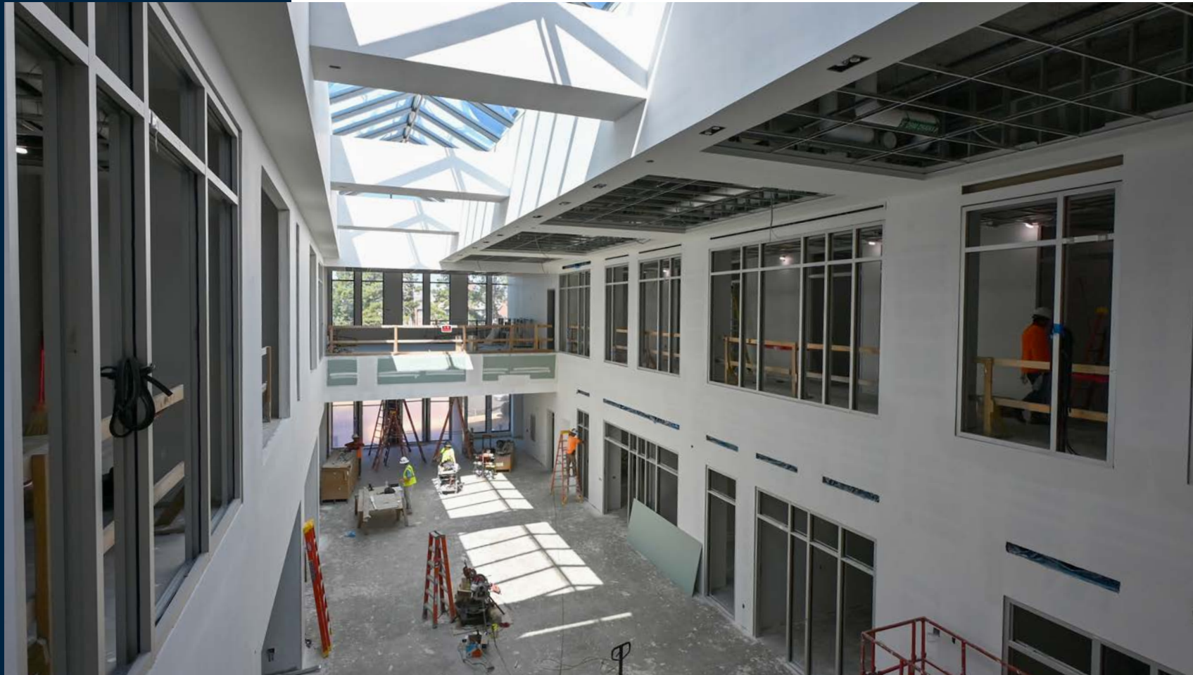
Drywall and interior window installation is complete in the central atrium space.
