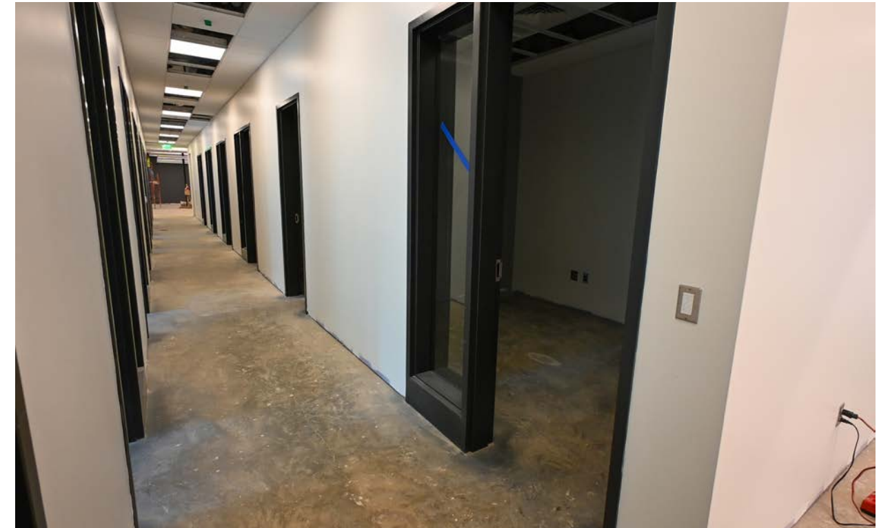
The offices are nearly complete with only a final coat of paint and flooring left to finish.
