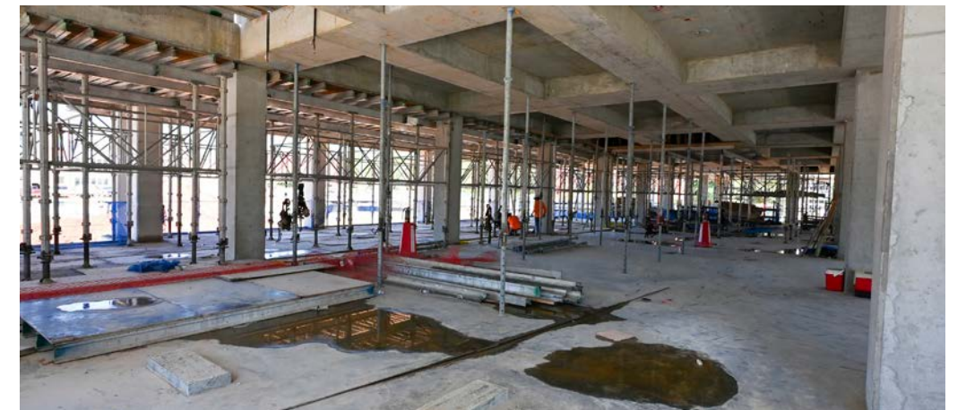
Internal support braces are being removed on the lower levels of Building B.
