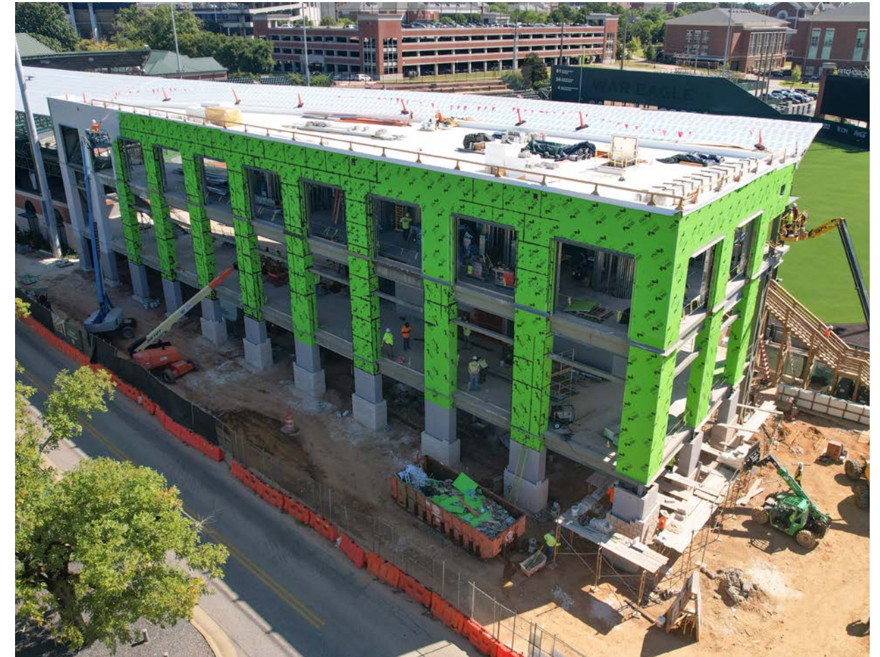
A green protective waterproof barrier has been installed and brick work will begin soon.
