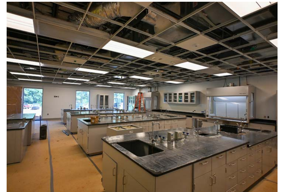
Fume hoods and lab casework have been installed with final gas, water and electrical lines to be connected.
