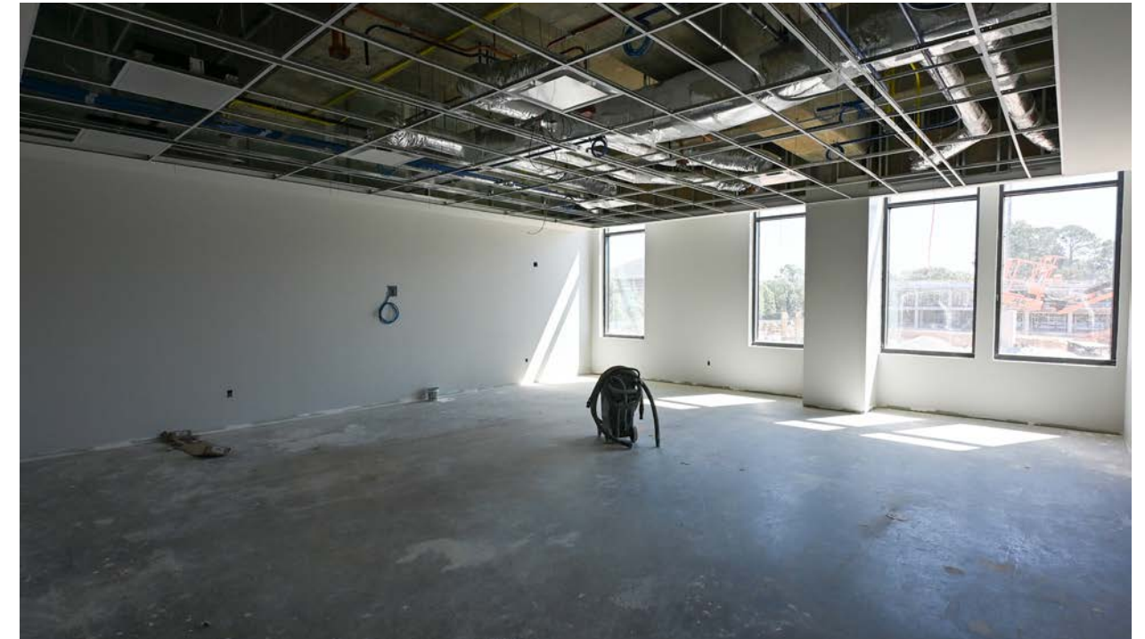
A computer lab on the second floor has been cleaned in preparation for ceiling tile and flooring.
