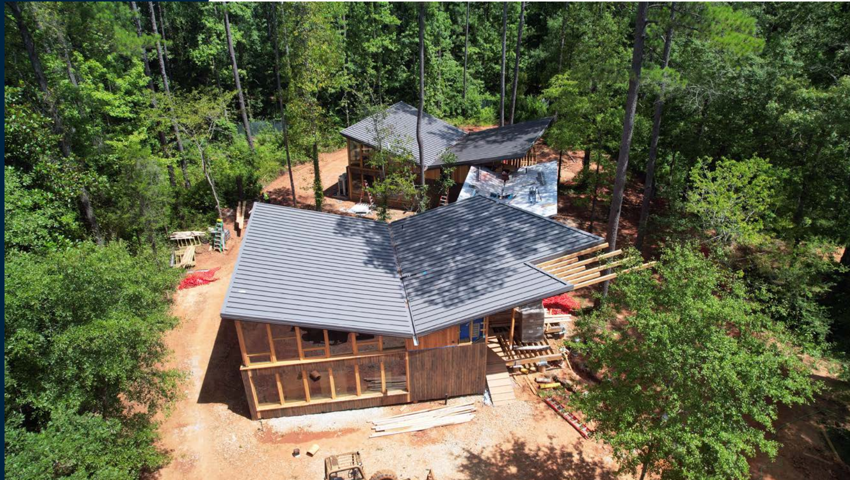
An aerial view of the Kreher education building shows work continuing on the main structures including siding and conditioning of the CLT structure.
