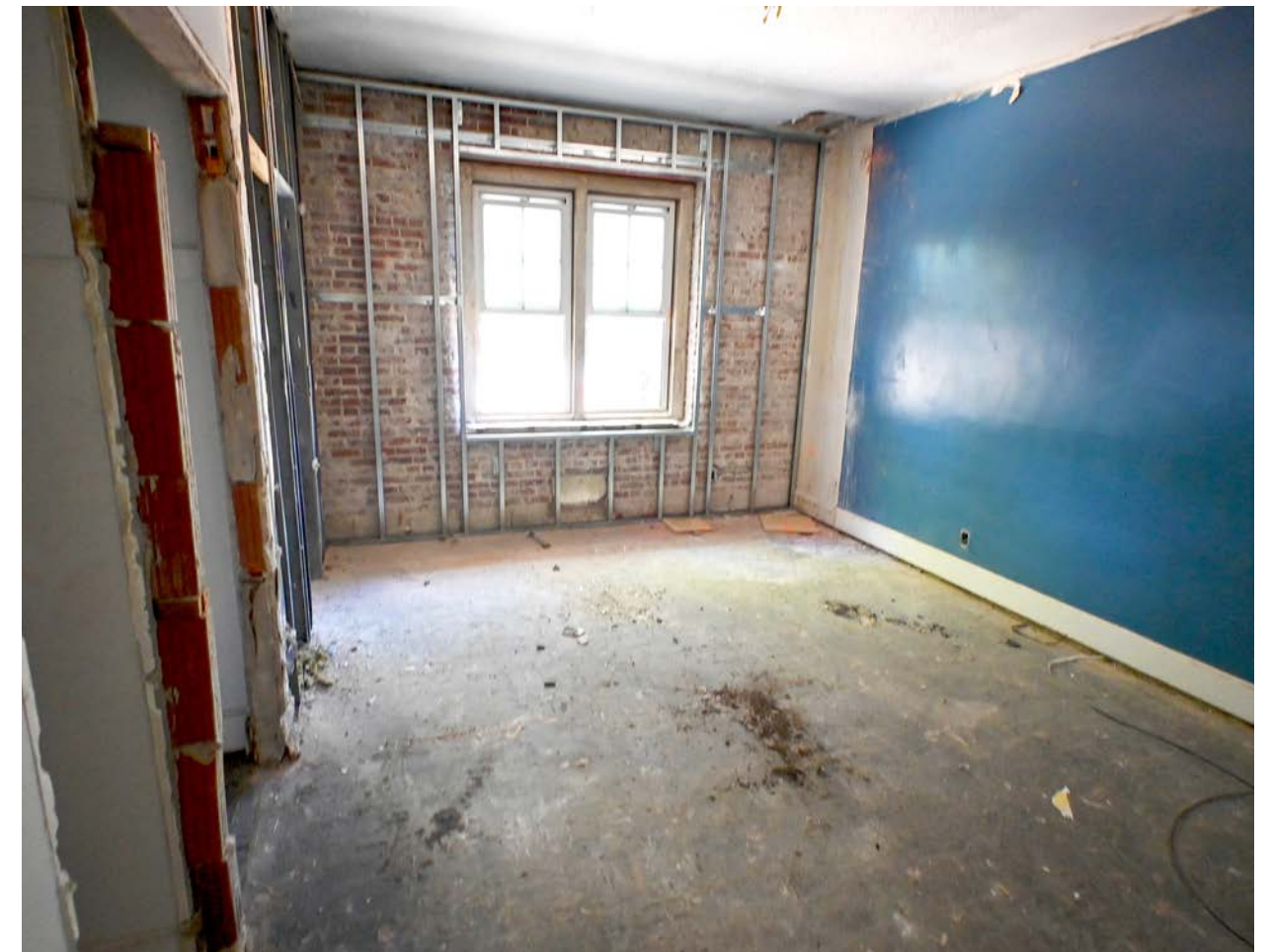
The finishes throughout all the bedrooms have been removed, preparing the area for upgrades.
