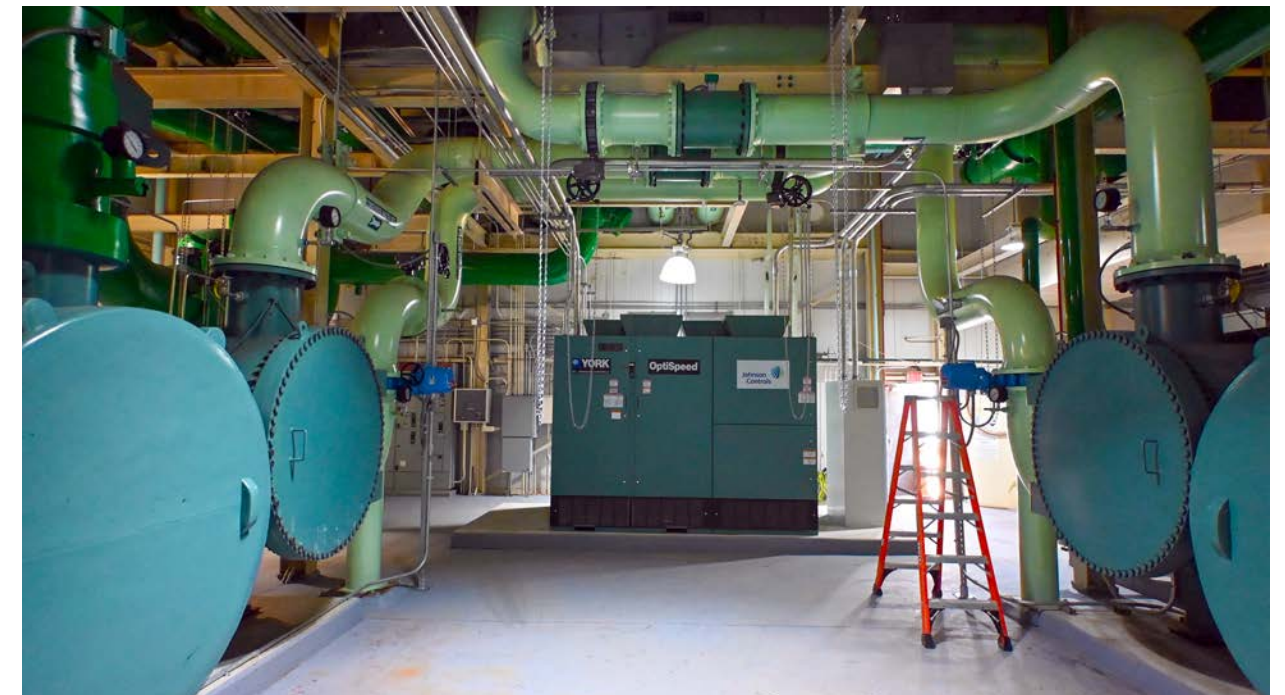
Far left and far right, the two new 1,600-ton chillers provide a more adequate amount of chilled water to be utilized by veterinary medicine in a more efficient capacity.
