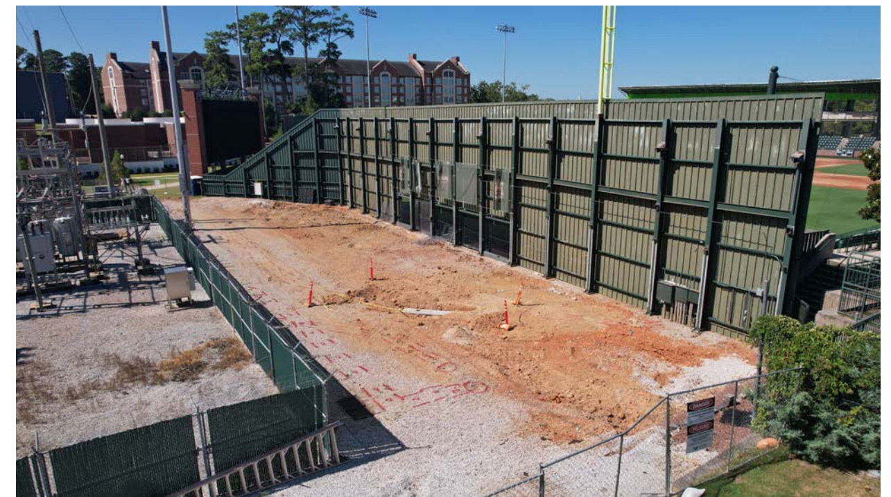
The bullpen has been demolished in preparation for the War Eagle Wall terrace.
