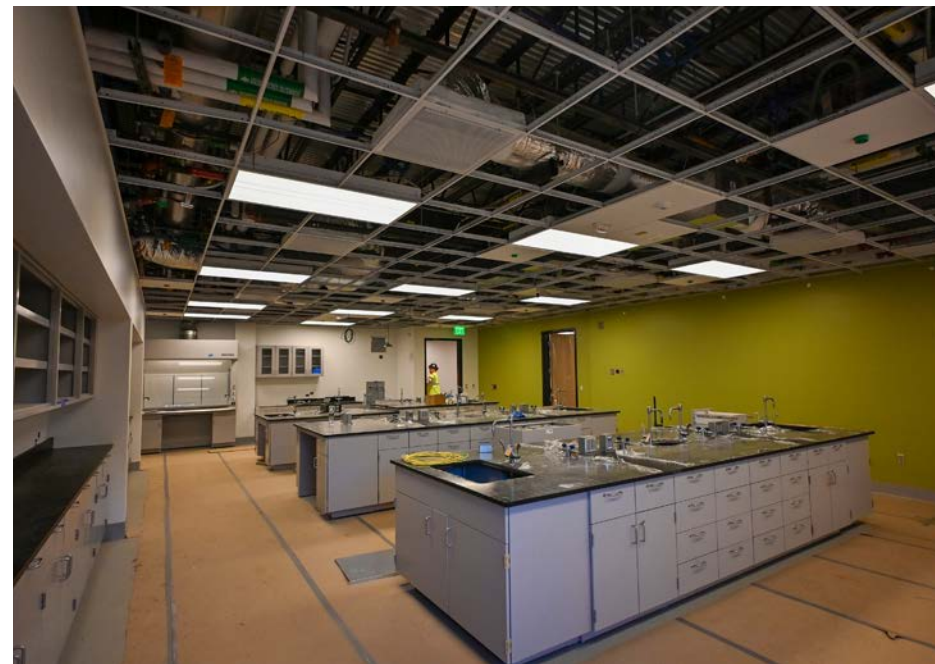
The finished floors remain covered while this lab awaits ceiling tile installation.
