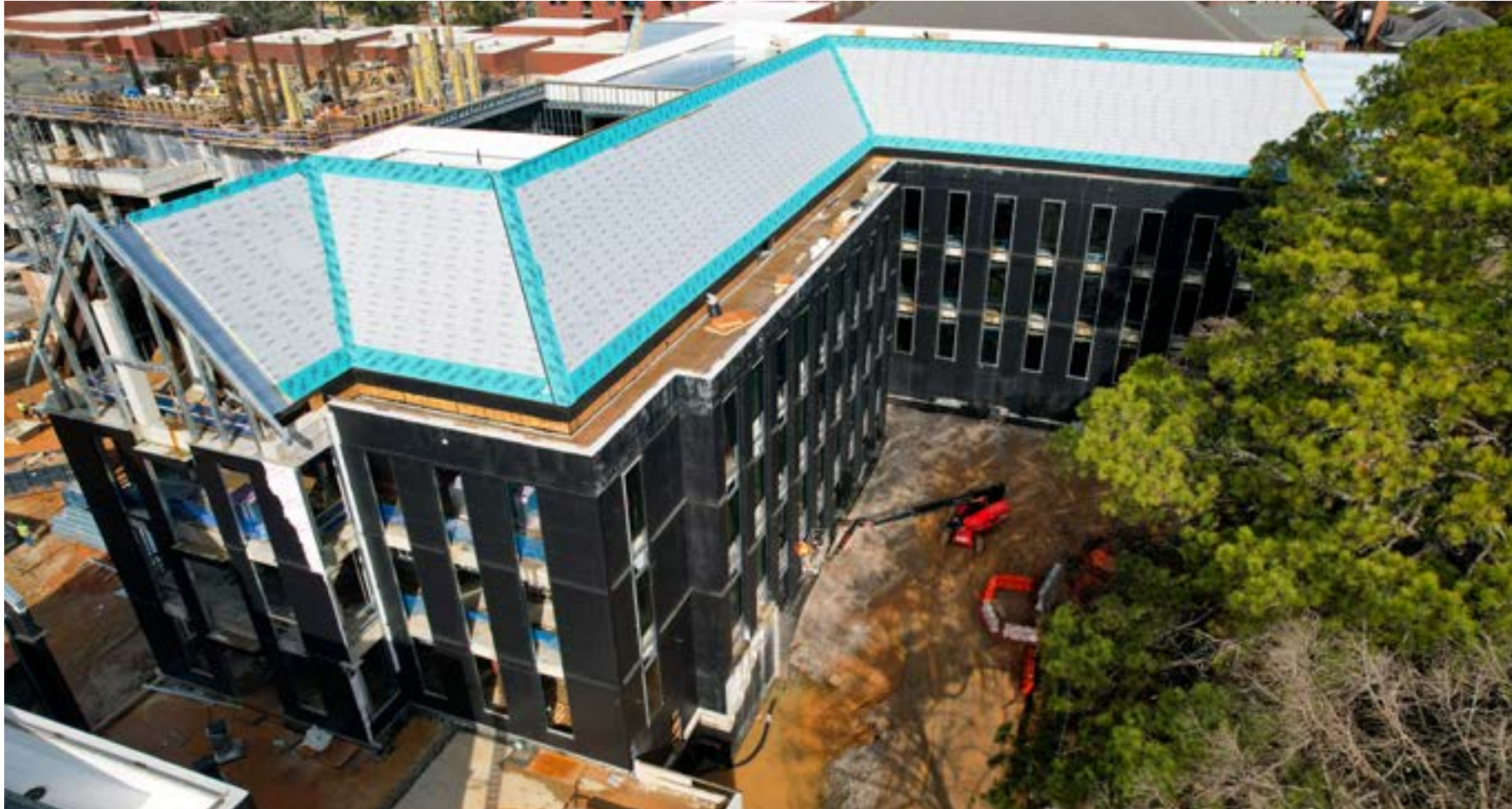
Roof framing and exterior sheathing are complete on Building B. Brick installation has begun at the basement level of the northeast side.
