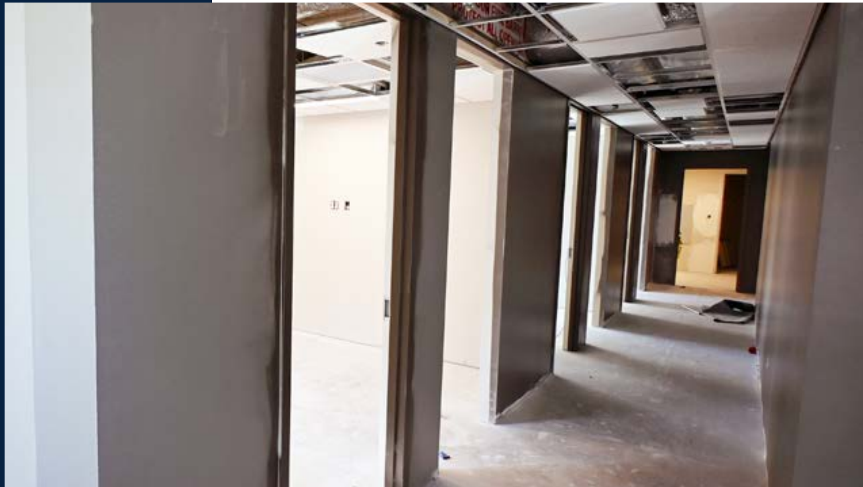
Offices have been painted and are awaiting installation of windows and doors.
