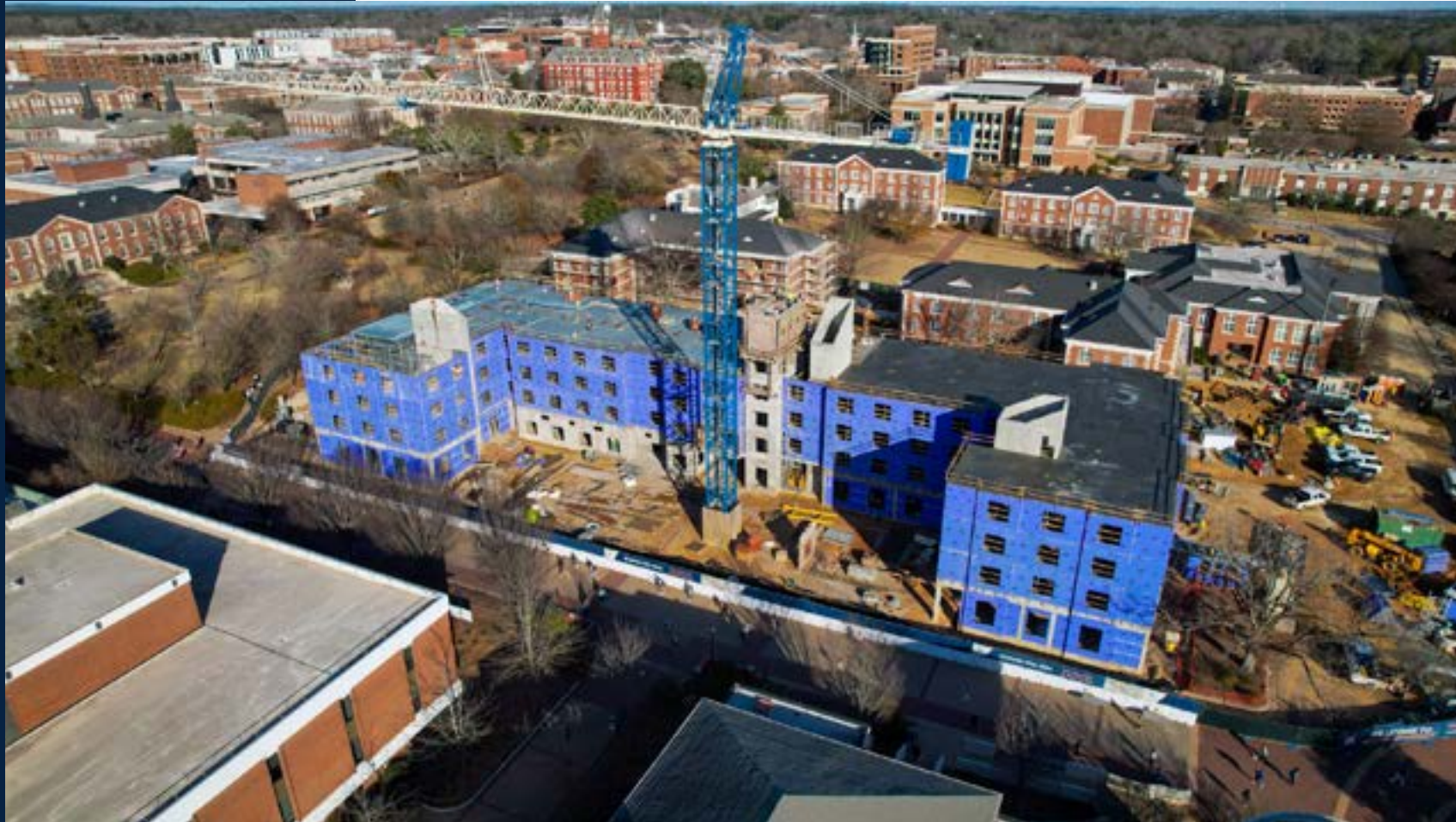
The exterior structure is nearing completion for the New University Student Housing project.
