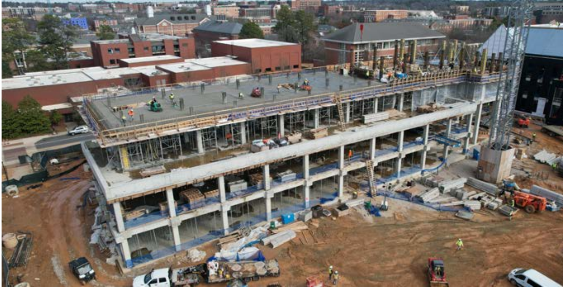
The remaining formation of Building A's concrete structure will be complete in early February.
