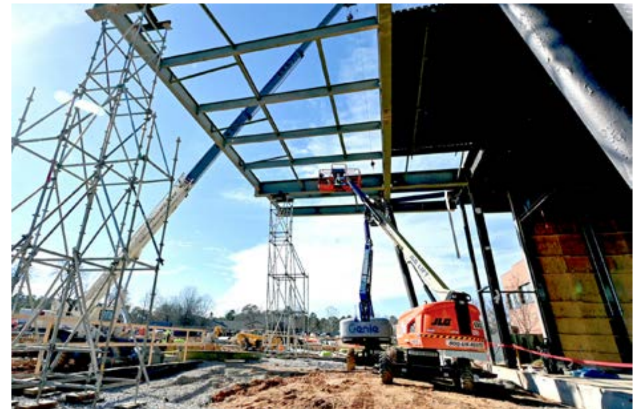
Structural steel is currently being positioned for extension of the outdoor stage canopy.
