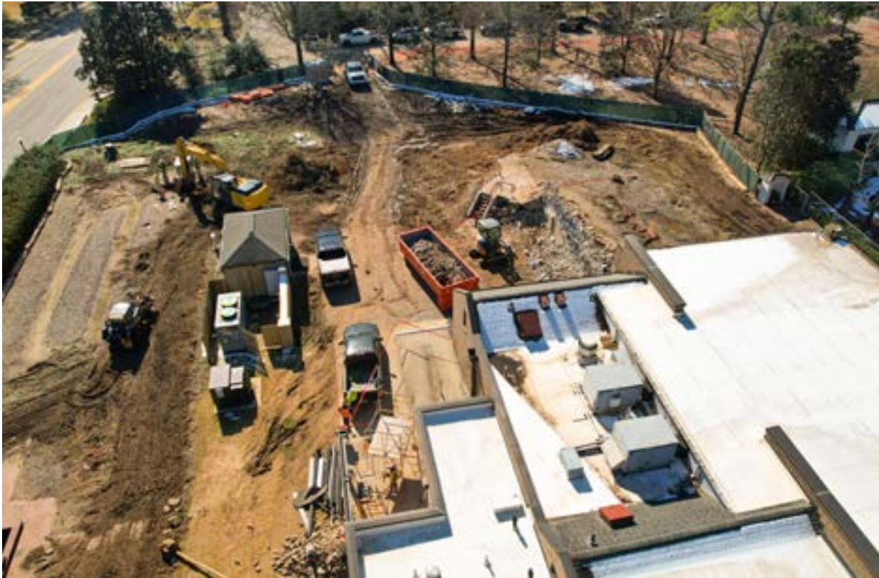
Removal of the temporary event tent is complete. Preparation for the installation of underground utilities has begun.
