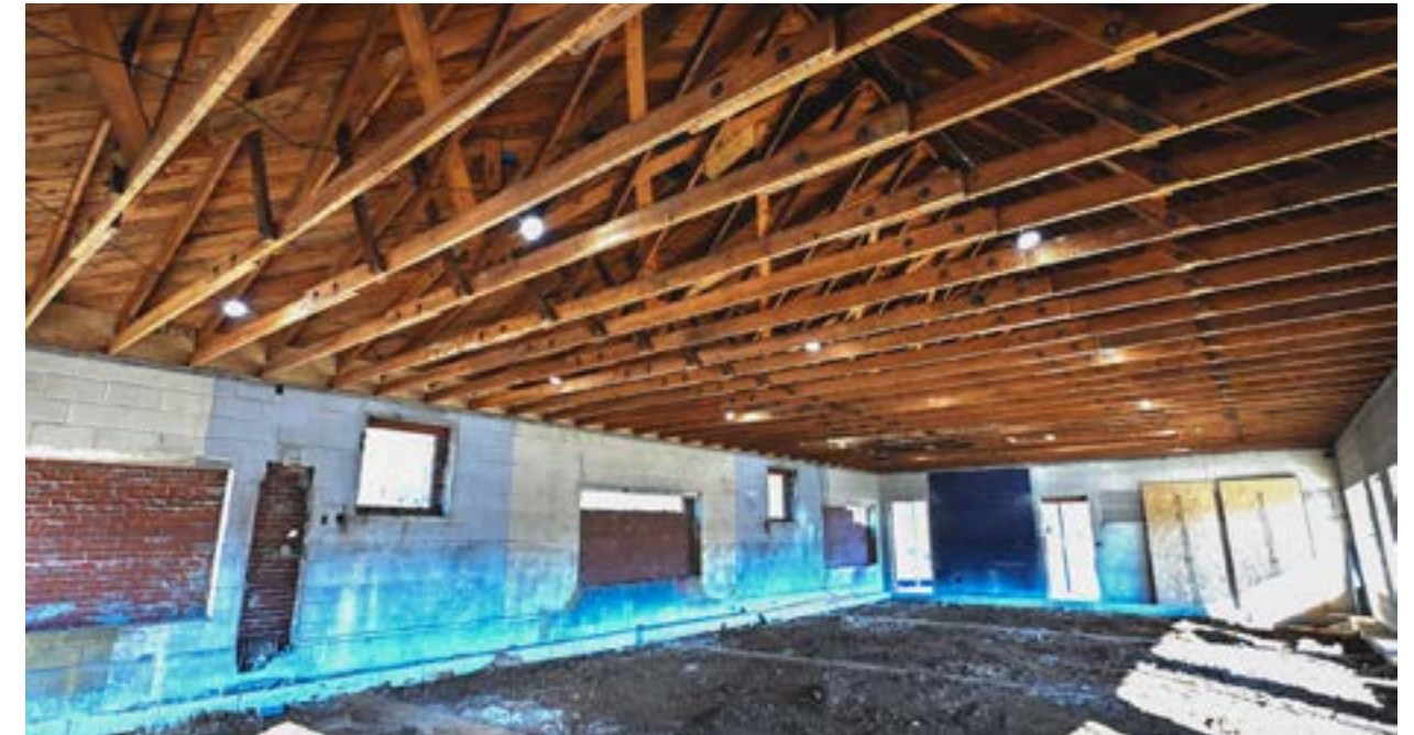
The interior infrastructure has been removed, making way for the installation of underground utilities.
