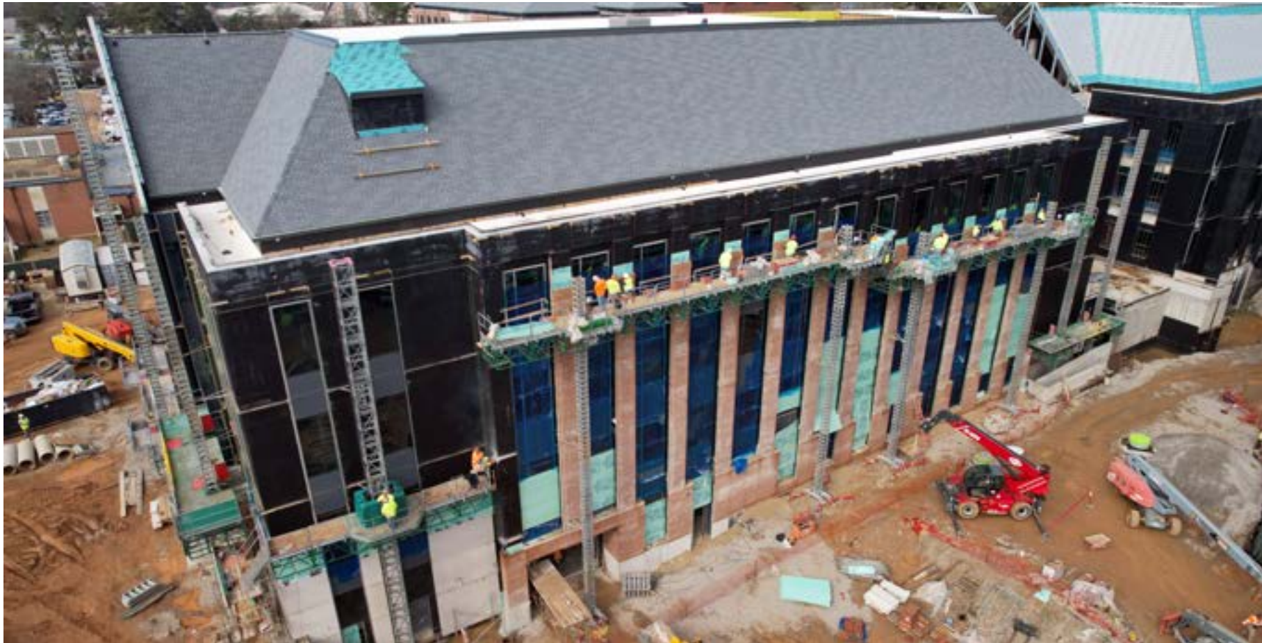
Progress continues on Building C as brick installation on the east side transforms the exterior, showcasing the structure's emerging design.
