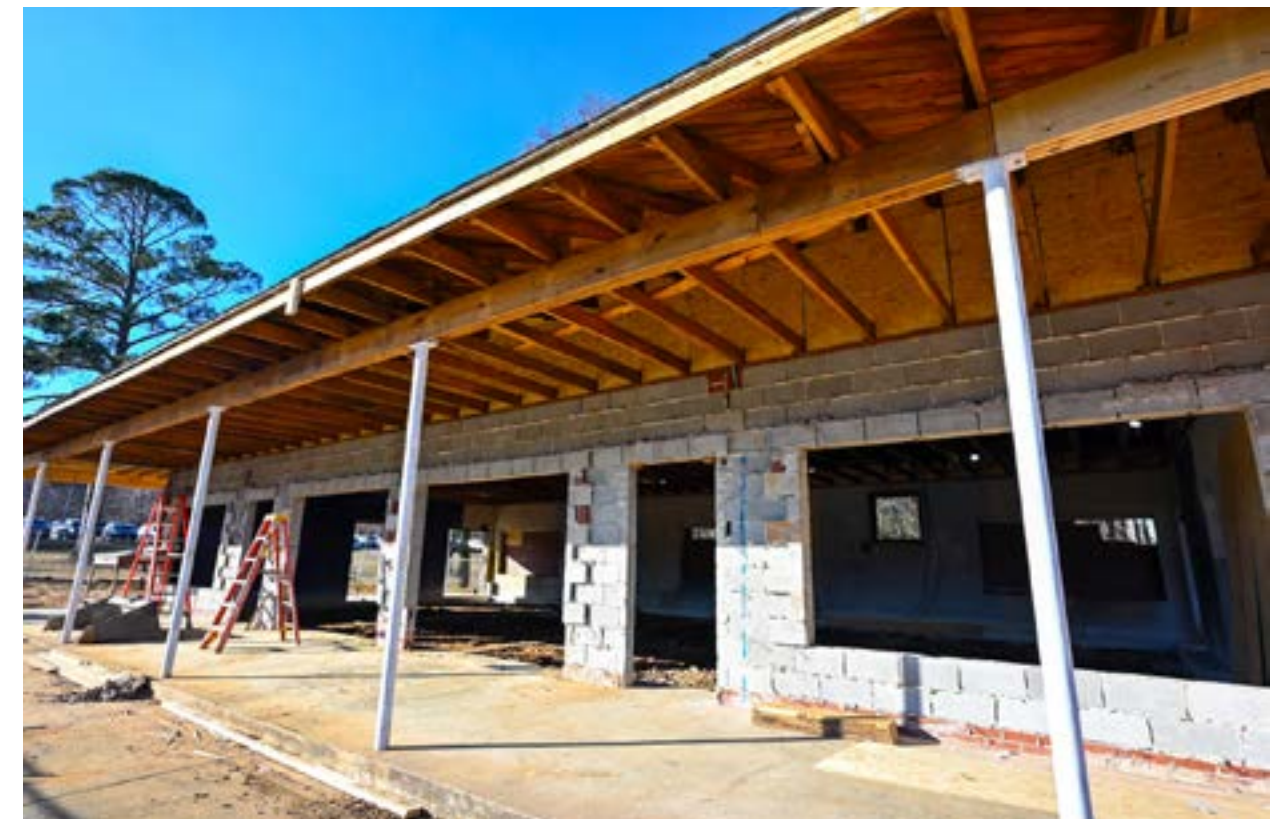
Demolition of the brick and other exterior building materials is complete in preparation of the building restoration.
