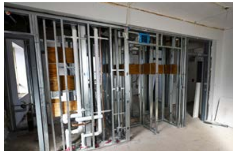
Mechanical, electrical and plumbing systems installation is taking place in the bathrooms of Teague Hall.
