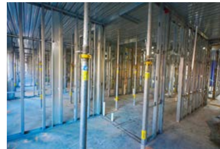
Installation of mechanical, electrical and plumbing systems has begun on the second floor.
