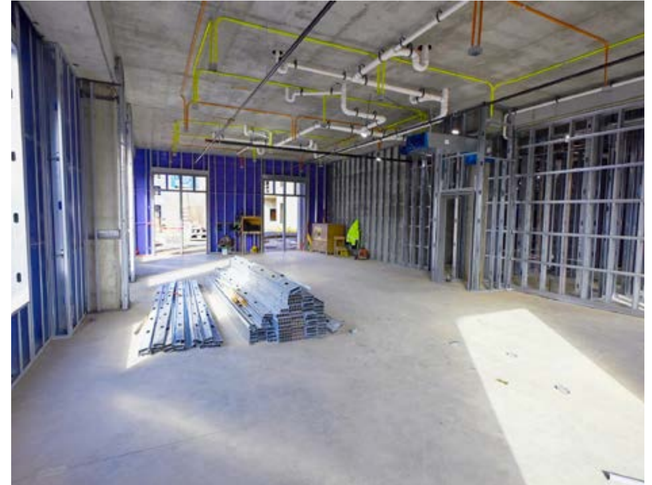
Installation of overhead mechanical, electrical, fire protection and plumbing systems is taking place in the student community room.
